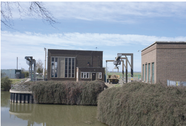
Pumping Stations at Pode Hole © Bob Harvey. Licensed for reuse under the Creative Commons Licence.
