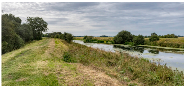
Raised embankments on the River Witham near Woodhall Spa © Julian P Guffogg. Licensed for reuse under the Creative Commons Licence.
