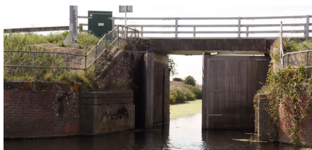
Sluice gate on the Timberland Delph © Chris. Licensed for reuse under the Creative Commons Licence.
