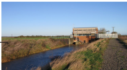
Black Hole Drove Pumping Station © Alex McGregor. Licensed for reuse under the Creative Commons Licence.
