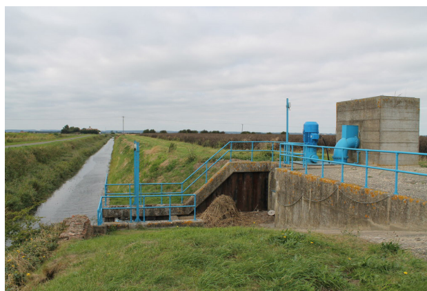
Haconby Fen Pumping Station © J.Hannan-Briggs. Licensed for reuse under the Creative Commons Licence.
