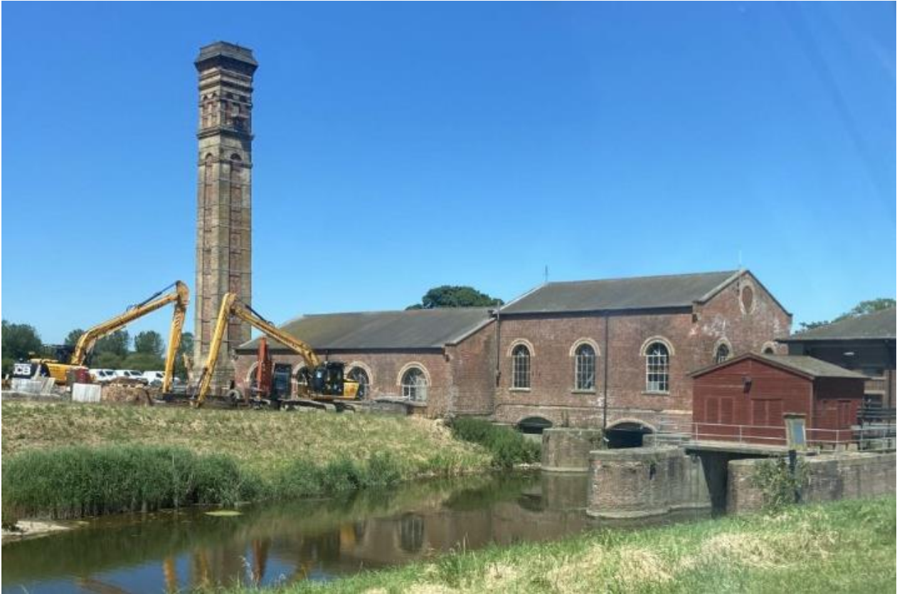
Figure 9: Lade Bank Pumping Station © Arup
