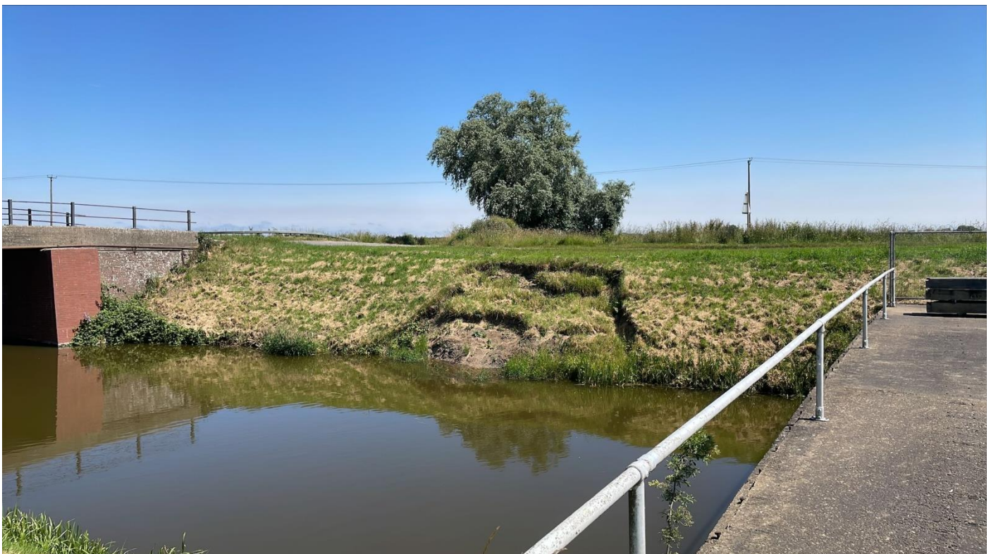
Figure 10: Photograph 1: Riverward collapse and slumping upstream of Lade Bank Pumping Station
