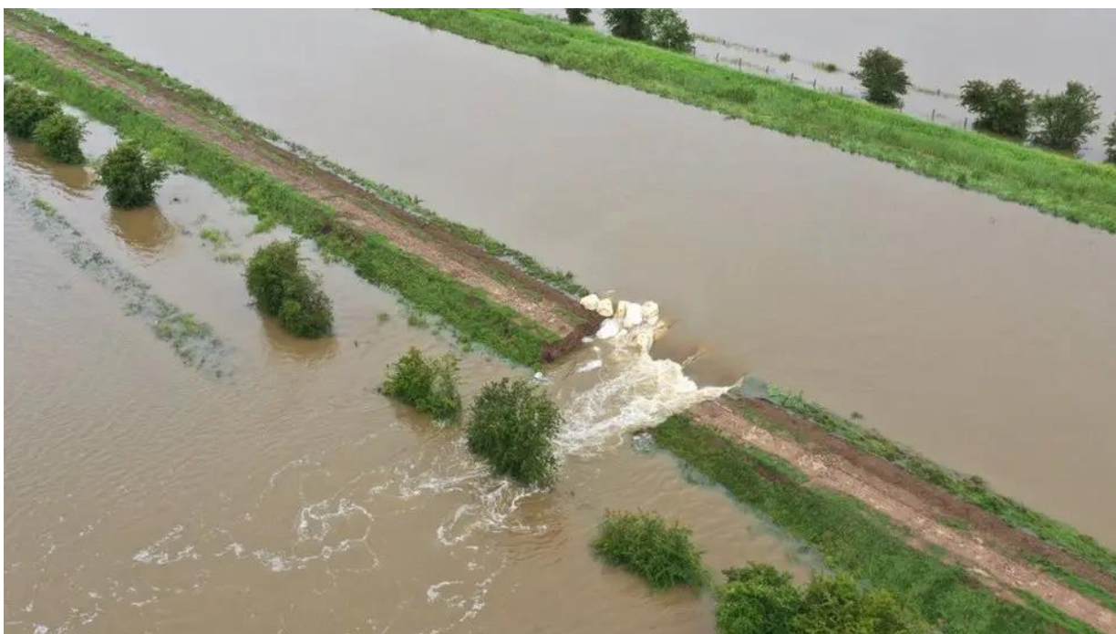
Figure 10: Breach in Relief Channel 22
