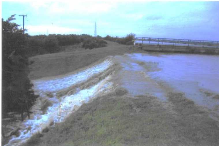
Figure 9: Images showing overtopping of the relief channel © Environment Agency
