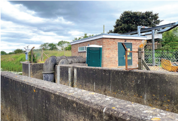
Croft Lane Pumping Station © Arup 2024
