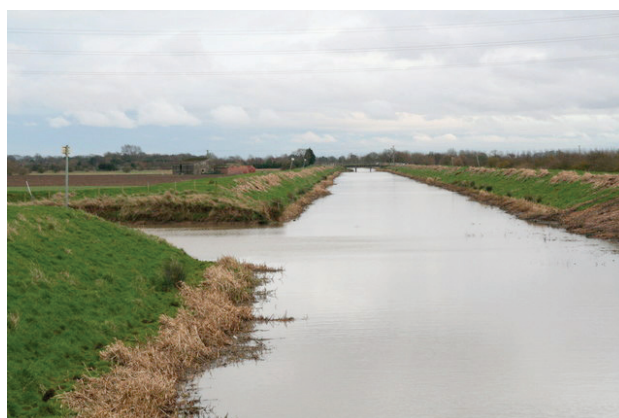
Wainfleet Relief Channel (left) splits from the Steeping River at Thorpe Culvert © Chris. Licensed for reuse under the Creative Commons Licence.
