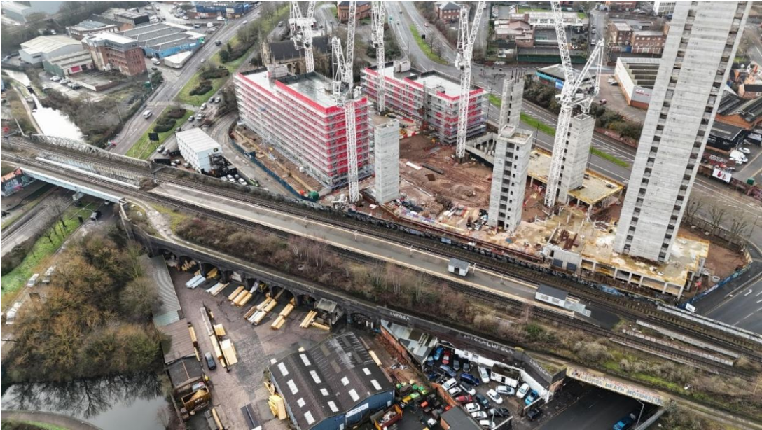
Figure 2: Bordesley station platform is in the centre of the picture. The Smith's Garden development currently under construction is at the top. The proposed site of the Bordesley West Chord is to the left of the development and the proposed site of the Bordesley East Chord is to the bottom left of the picture.
