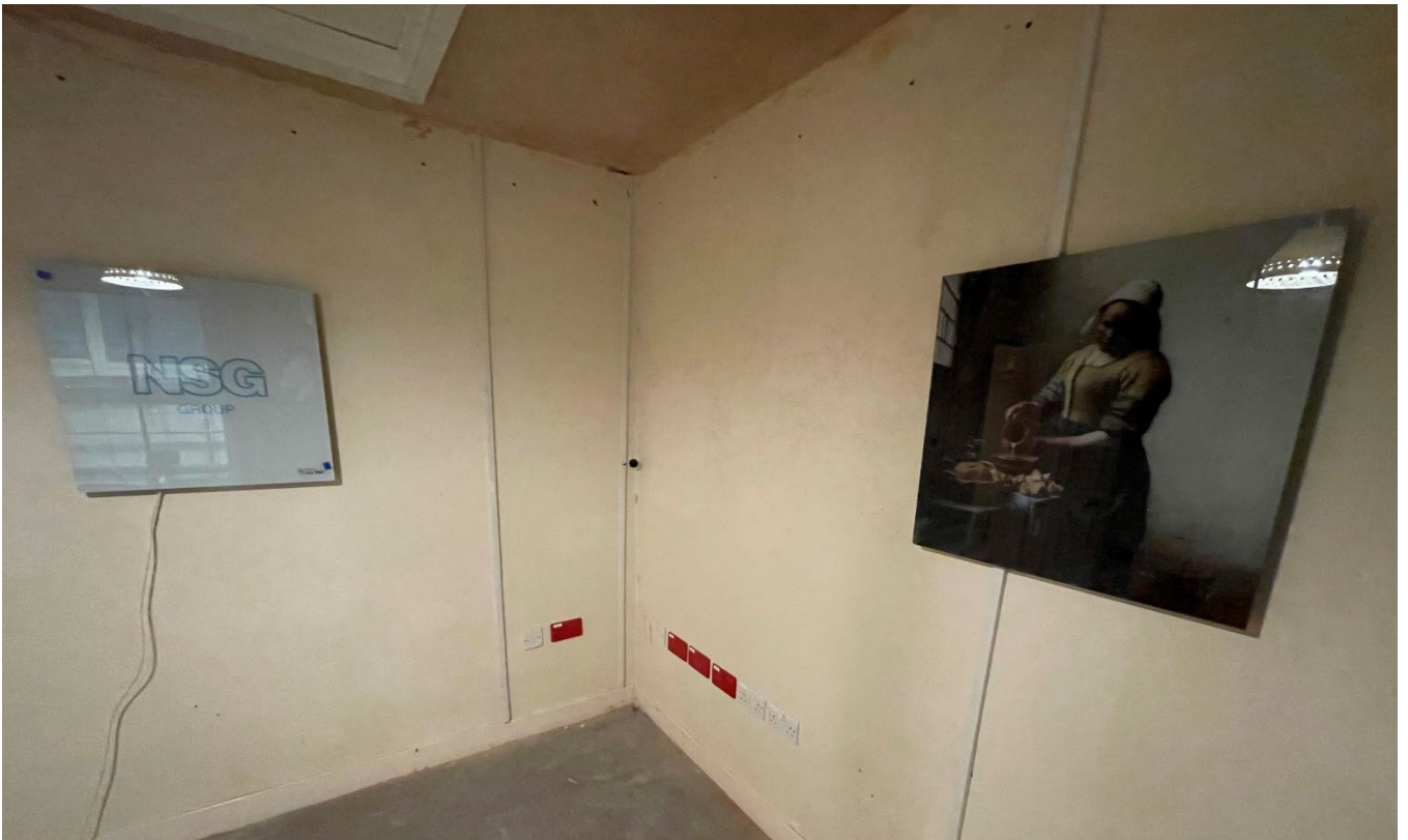
Figure 2-7 IR Heater type 4 installed in Room C
