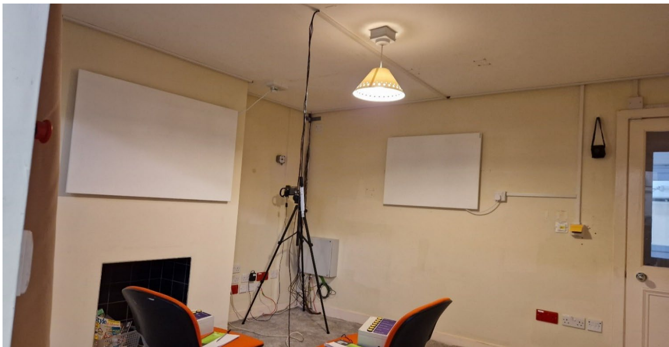
Figure 2-5 IR Heater type 1 installed in Room B
