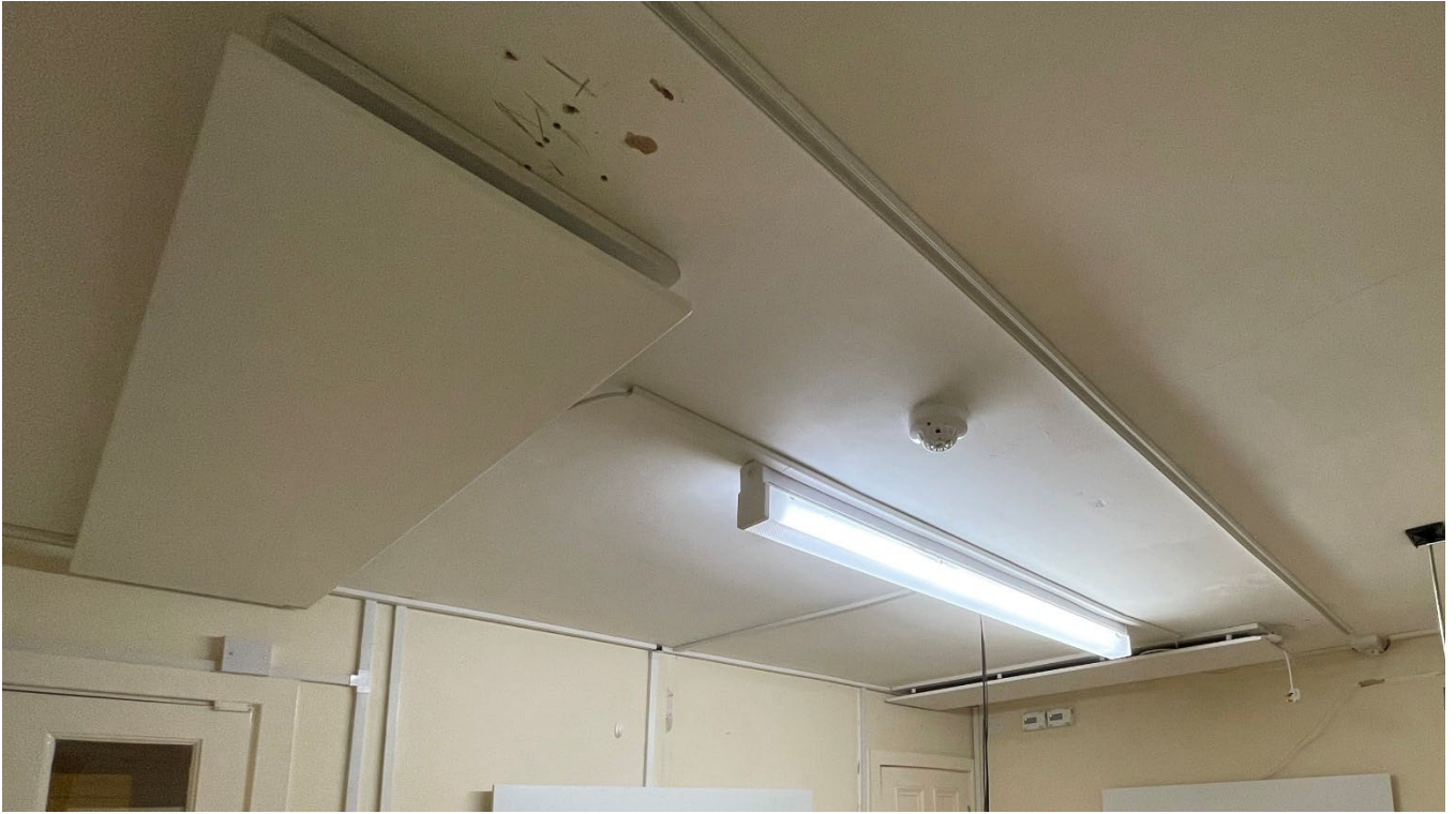
Figure 2-6 IR Heater type 2 installed in Room A
