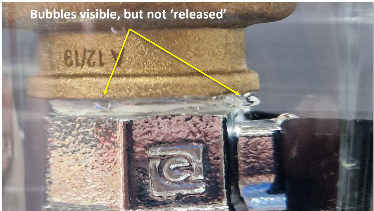
Figure 23: Observing bubbles from submerged valve connection on string 2303
