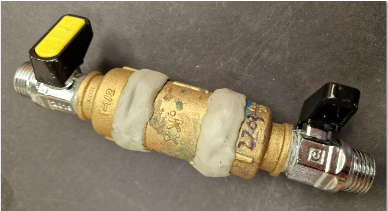
Figure 29: Temporary external wrapping on leaky string 2203
