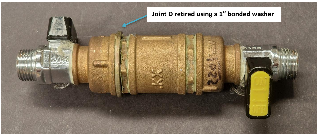
Figure 44: String 2201 after final leak test, with joint D retired
