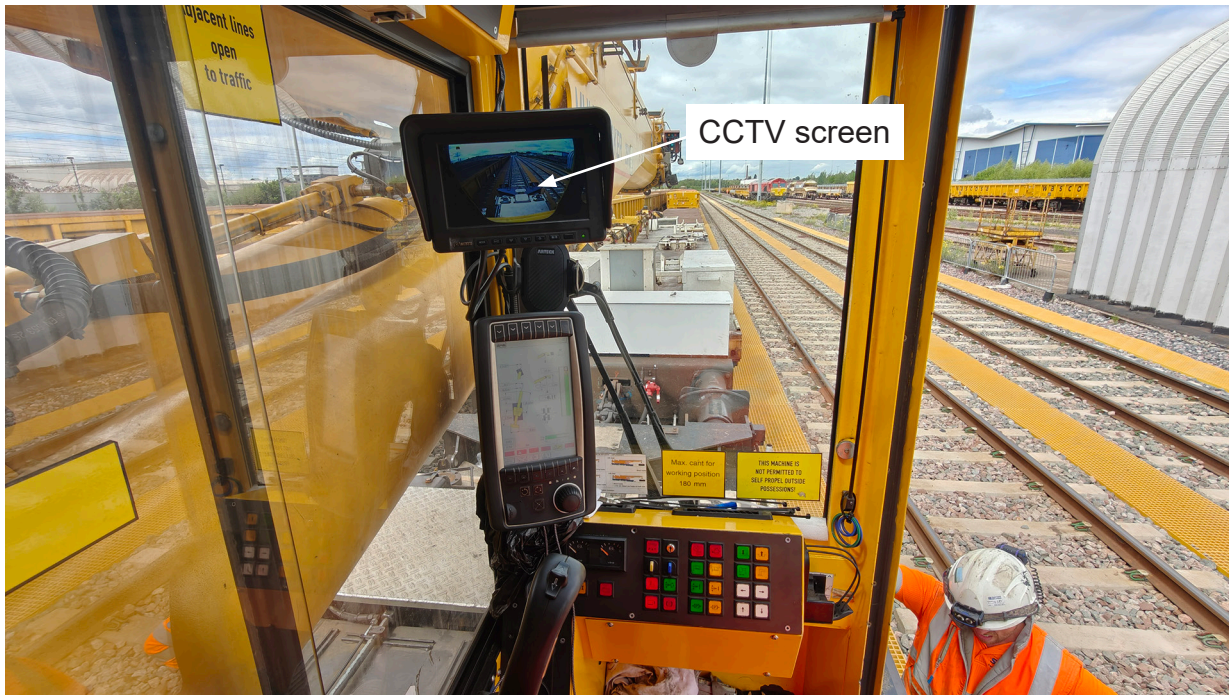
Figure 11: CCTV screen in cab of crane 26.
