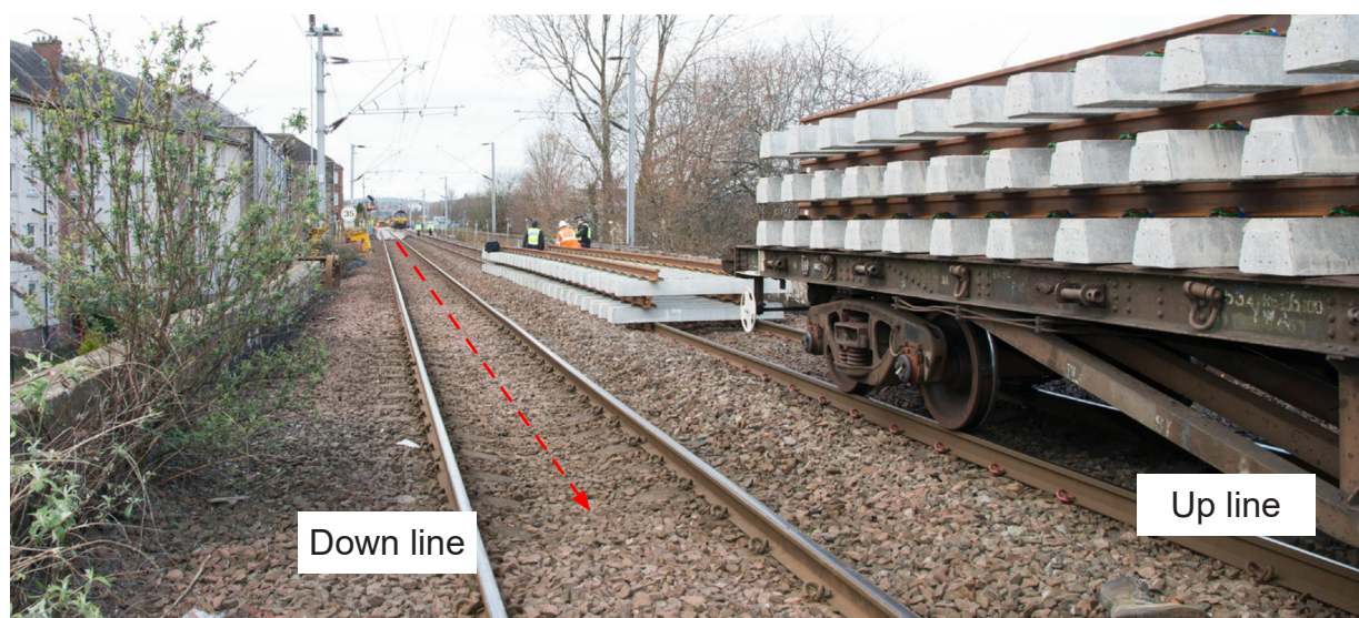
Figure 14: Walking route of the crane 26 controller on the approach to the accident (courtesy of British Transport Police).
