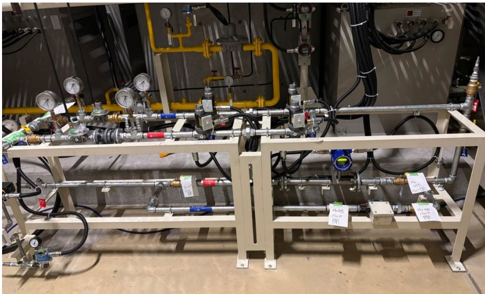
Figure 29 - Hydrogen Burner control system
