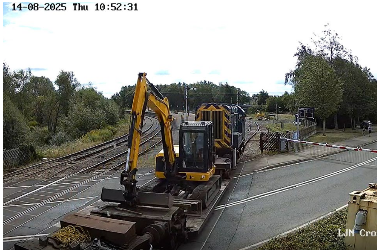
CCTV image showing incident train travelling towards the camera near Lydney Junction station, shortly before the accident (courtesy of Dean Forest Railway).
