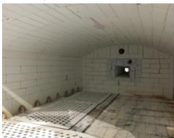
Figure 6: Photo of Glass Futures' CTB interior, viewing the rear furnace wall from the opened back wall end
