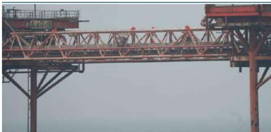
Photograph 9. Faecal staining on platform walkway of Inde 18A.
