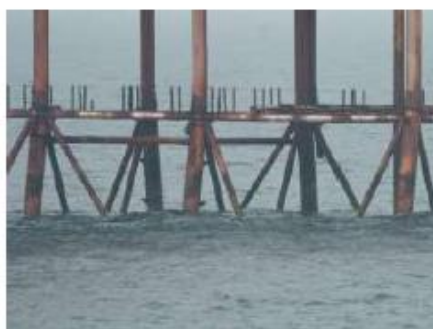
Photograph 8. Faecal staining on platform frame on Inde 18A.
