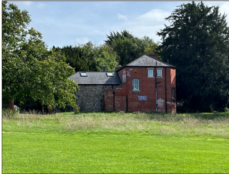
Image 15: Graffiti on wall of Listed Building
