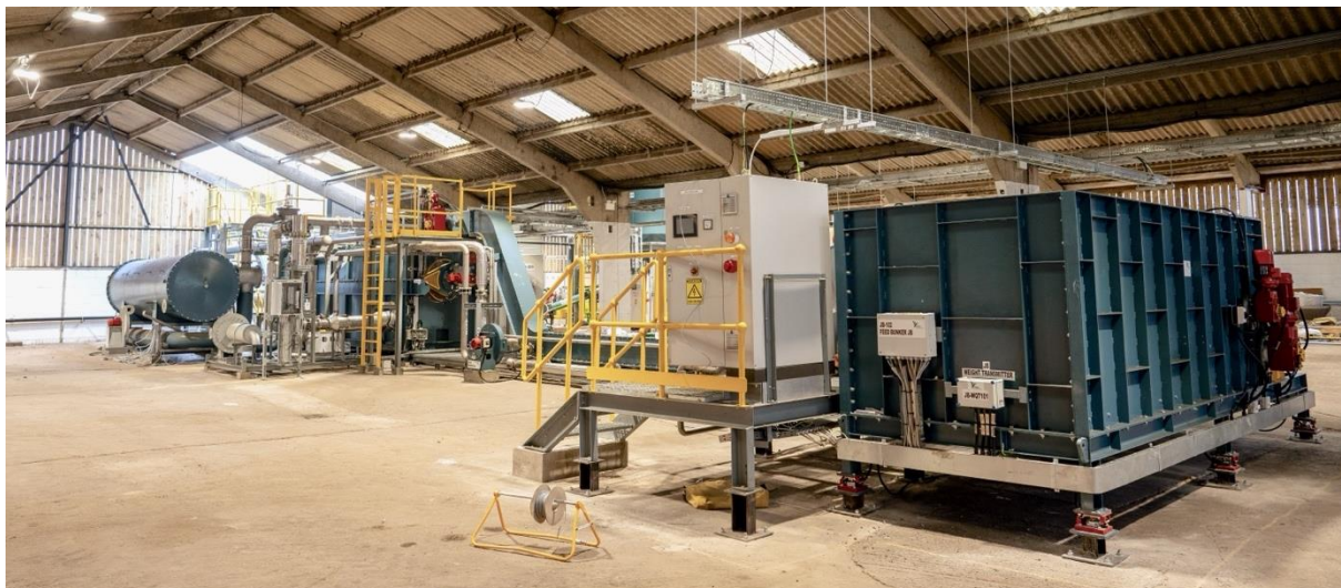
Figure 1.2. Lapwing Energy's Pyrolysis Plant
