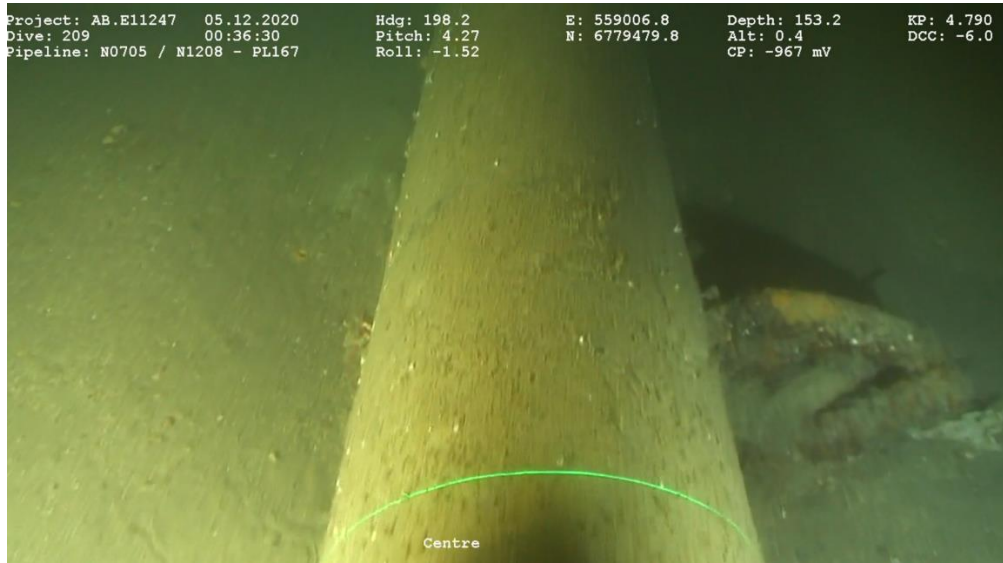
Figure 15-3 Pipe-in-pipe carrier pipe showing redundant trim chain (right hand side)
