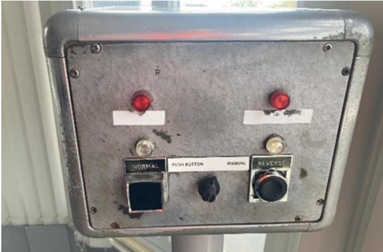
Figure 9: Redcar level crossing gates controls at the pedestal.
