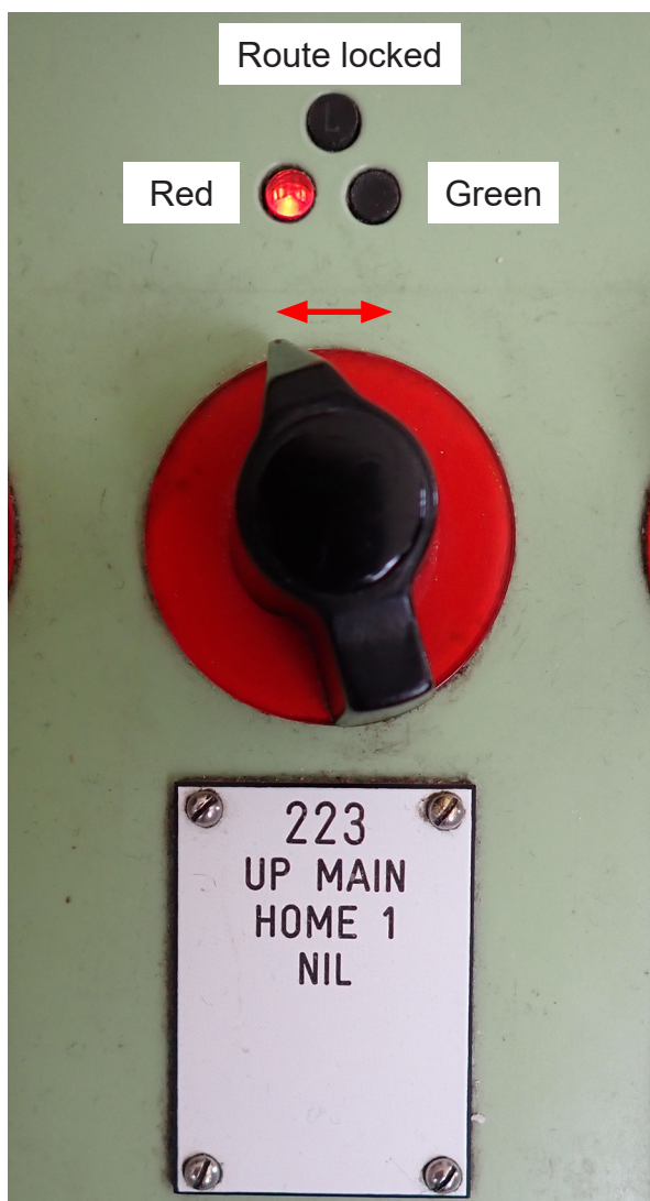
Figure 7: Signal R223 control on the Redcar signalling panel.
