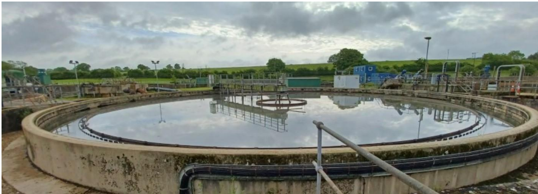
Figure A12-4 – Primary Settlement Tank at Chippenham WRC
