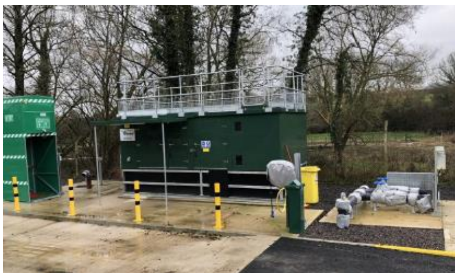
Figure A12-9 – Phosphorus removal assets at a WRC – Chemical dosing kiosk, emergency shower and bunded delivery area
