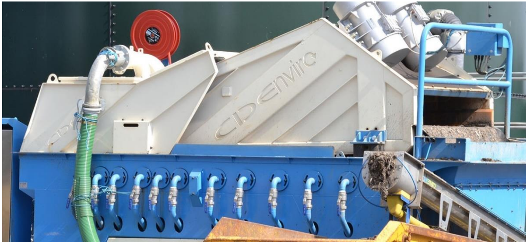
Figure A12-2 – Example of a sludge screen at Trowbridge WRC.
