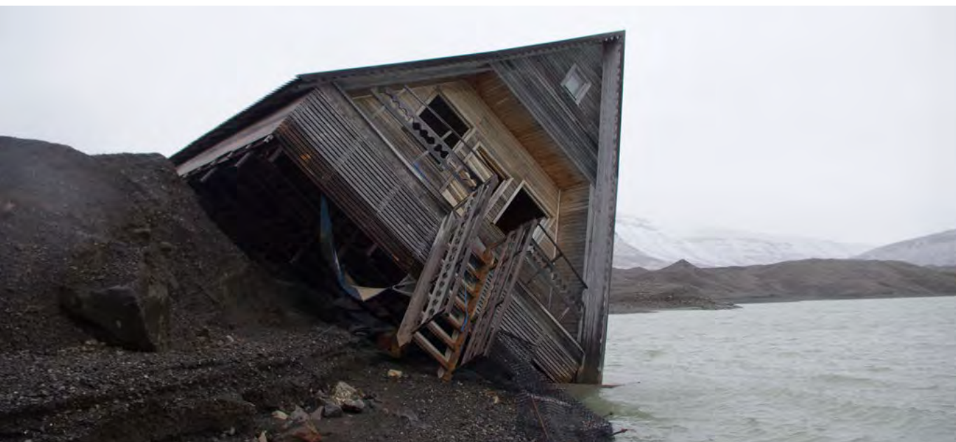
Temperature rises in the region are affecting the previously stable foundations of houses and other infrastructure
