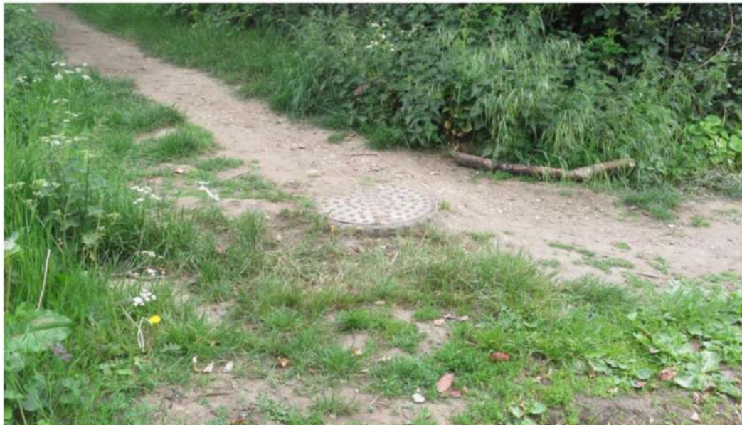
Photo 1: High stats cover in the public footpath
