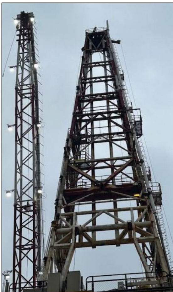
Figure 2.2: General view of Gannet A Mast with the west crane alongside the Crown
