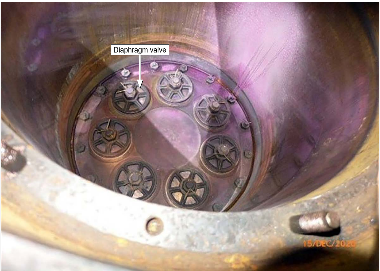
Figure 12: Vacuum pump diaphragm valves
