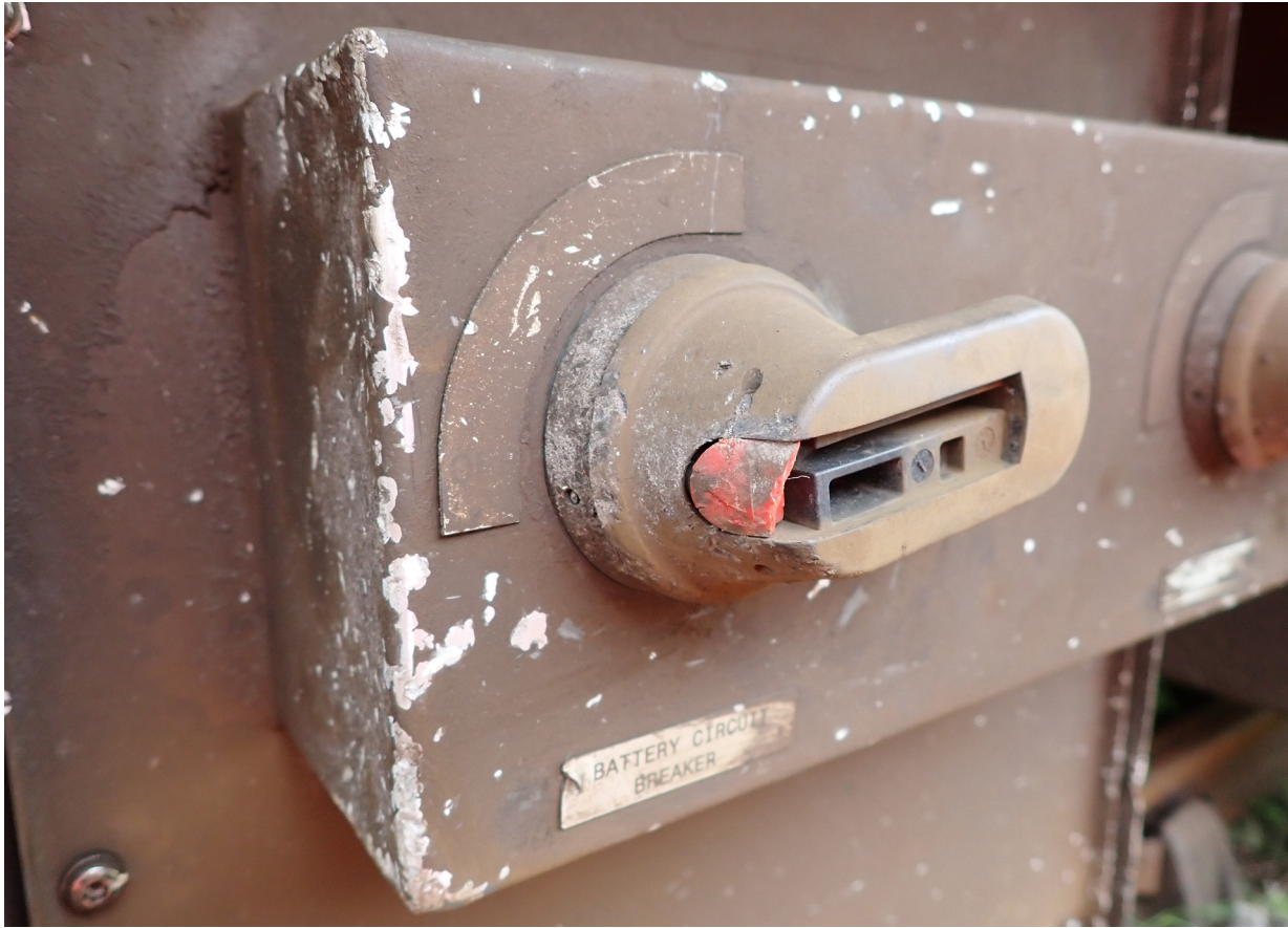
Figure 17: Damage caused to the battery isolation switch as it was knocked to the isolated position during the derailment.
