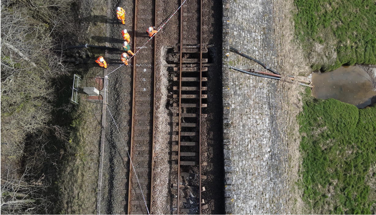
Figure 14: Overview of the site captured by a drone showing the adjacent line marked with a 3-2-1 countdown (courtesy of Network Rail).
