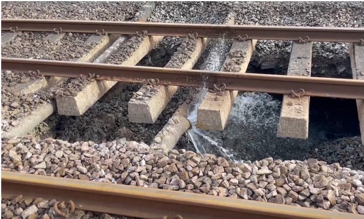
Figure 11: Water being sprayed from the damaged pipe during a site test.
