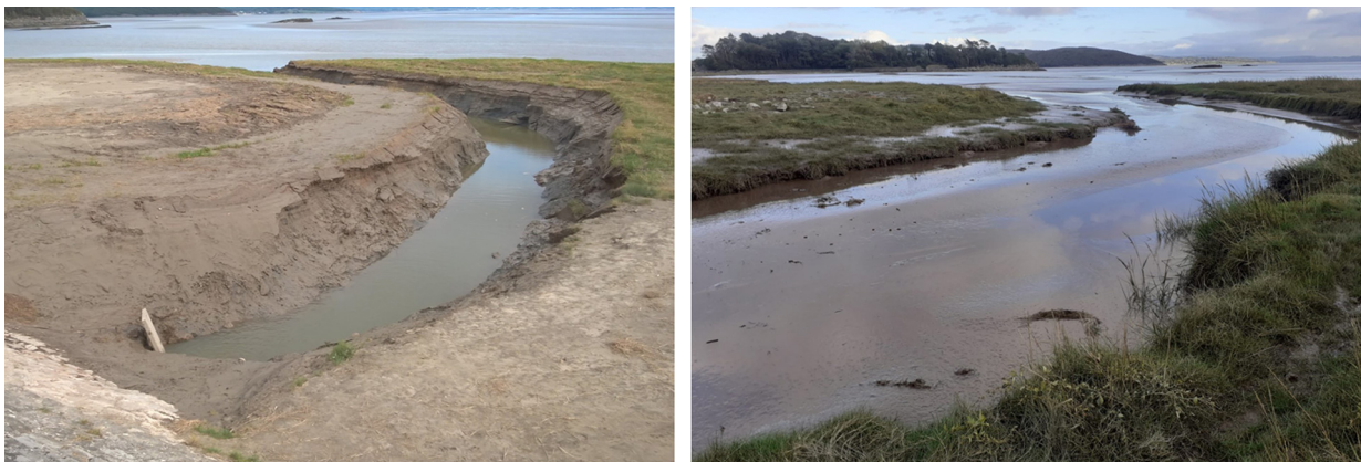
Figure 8: The outfall to Seldom Seen culvert pictured 3 to 4 months apart around May to September 2020 (courtesy of Westmorland and Furness Council).
