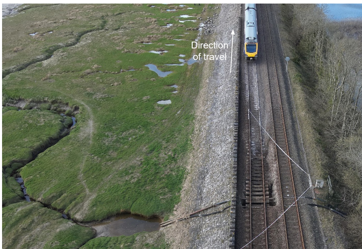
Figure 10: Void which opened under the track as train 2C37 passed (courtesy of Network Rail with RAIB annotations).
