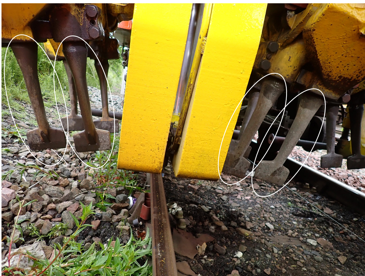
Figure 5: Tamper tines (circled) on the tamper involved in the accident.
