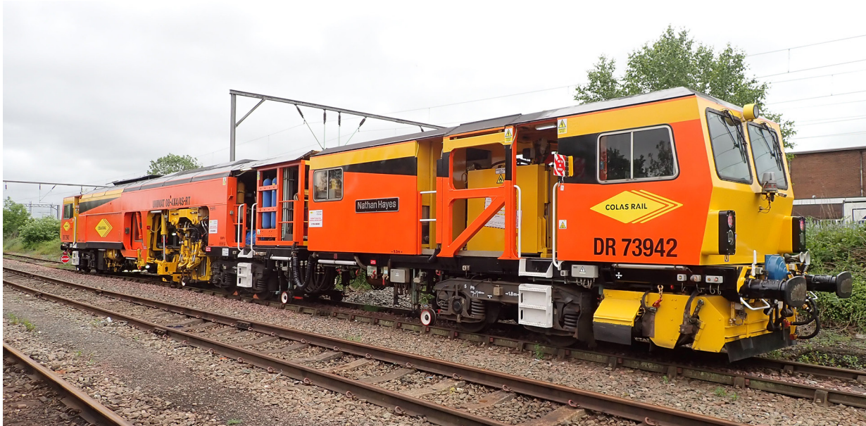
Figure 6: Tamper 6J87 which struck the pipe.
