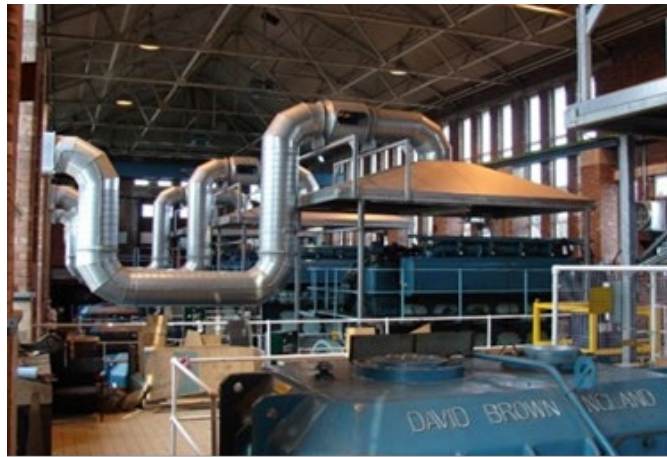
Figure 9.6 Inside the Black Sluice pumping station, Boston, Lincolnshire
