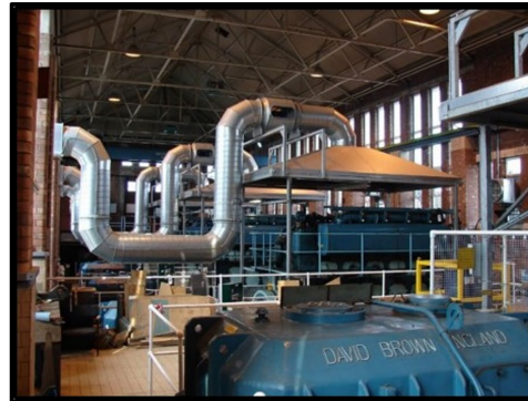
Pumping station and pumps
