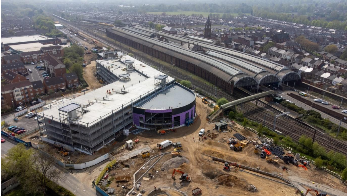
Aerial image of the multi-storey car park and station building in the centre left of the picture, with the transport interchange and short-stay parking to the bottom right. The area for the new platforms is just visible above the building.
