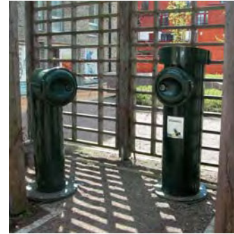
Image 79 Domestic waste chutes to underground storage, Malmö
