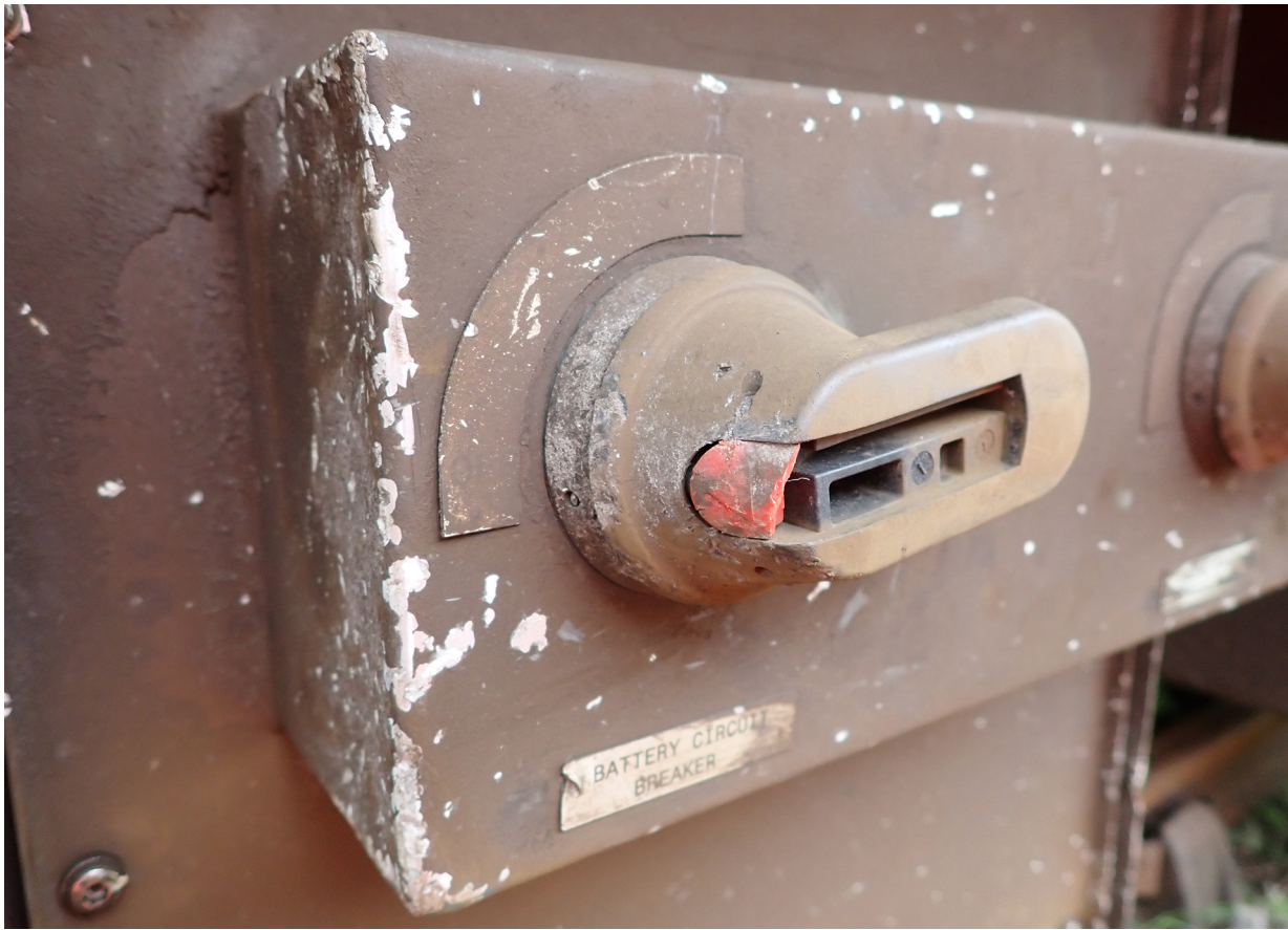
Figure 17: Damage caused to the battery isolation switch as it was knocked to the isolated position during the derailment.
