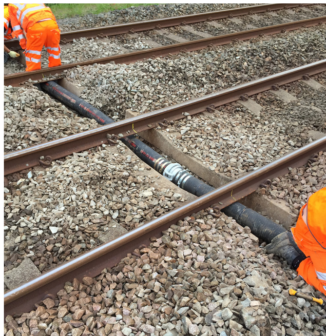
Figure 13: Installation of the pipe which was struck by the tamper (courtesy of Network Rail).
