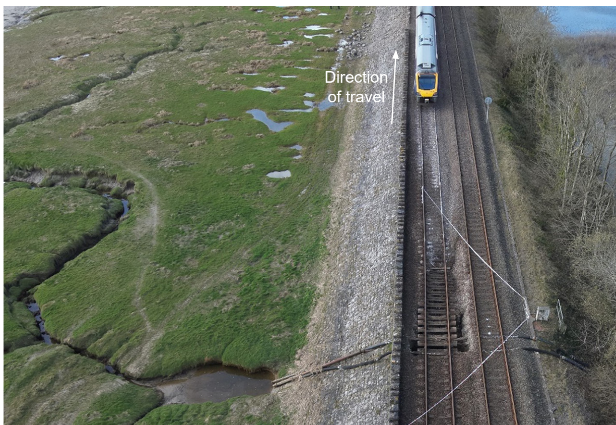
Figure 10: Void which opened under the track as train 2C37 passed (courtesy of Network Rail, with RAIB annotations).
