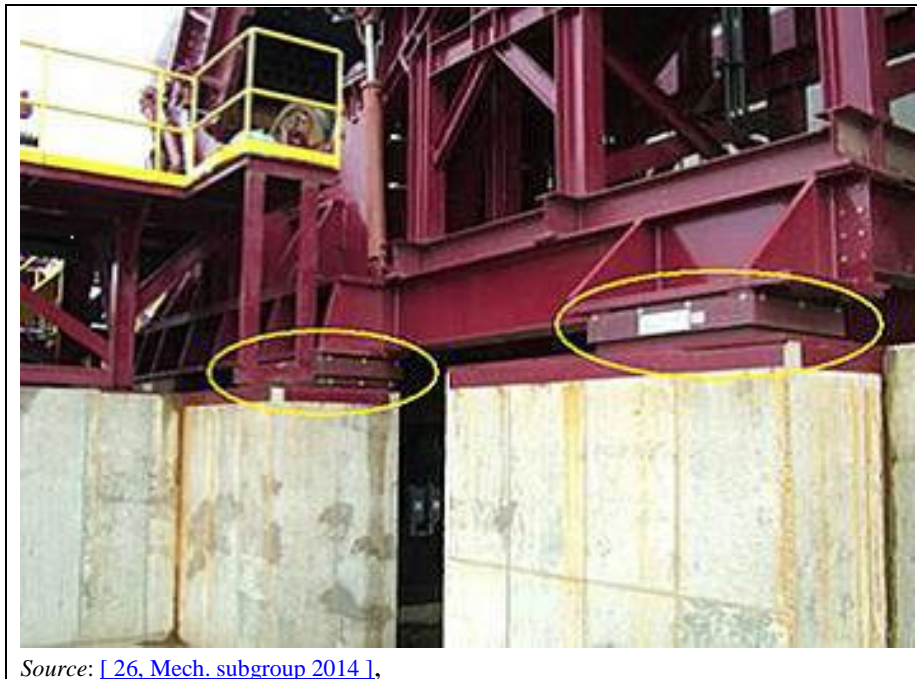
Figure 3.22: Isolation elements (circled) for vibration reduction
