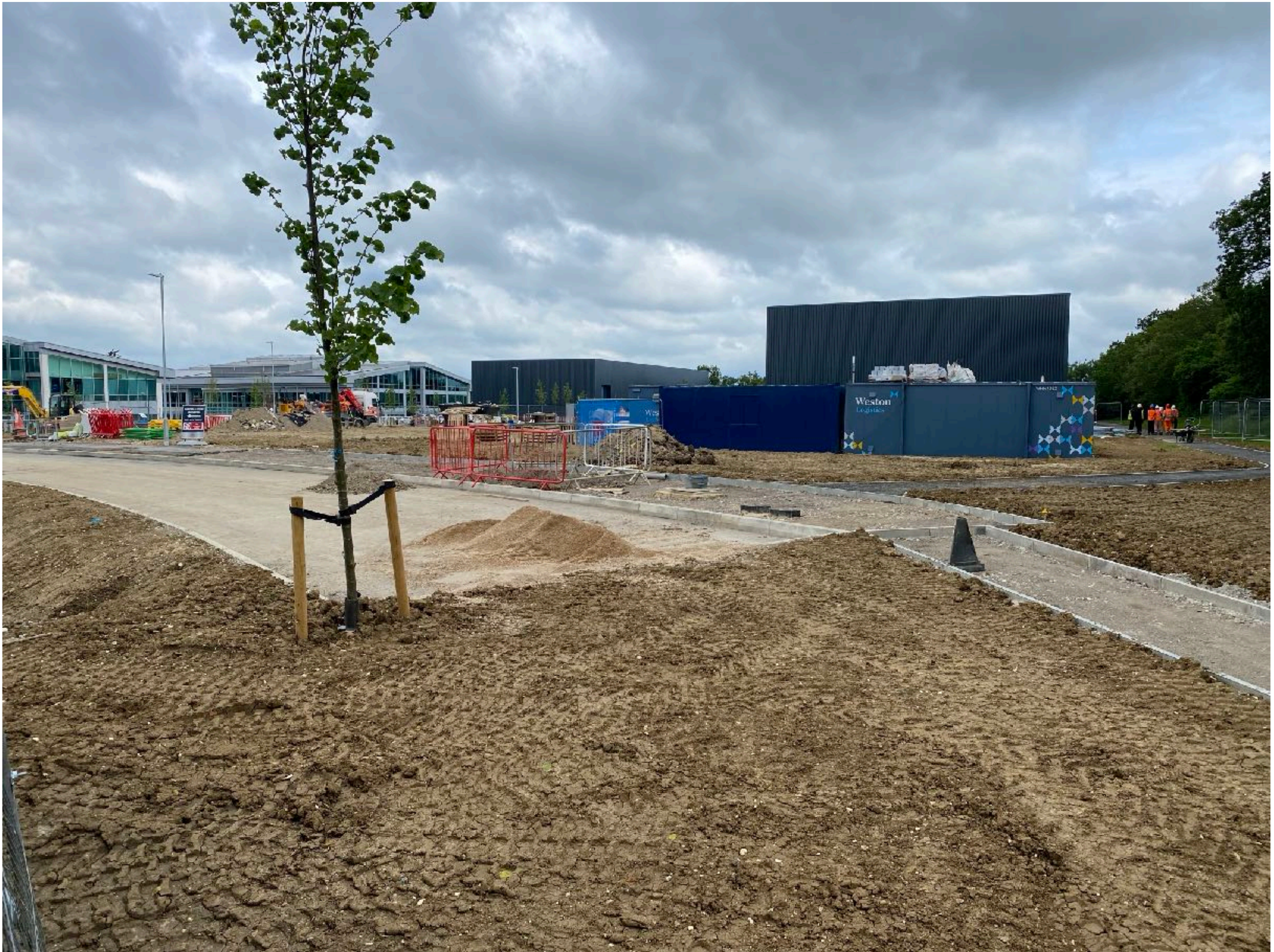
Photo 4: Completed roadway running to SW corner of Priors Wood which was never shown on approved planning documents.
