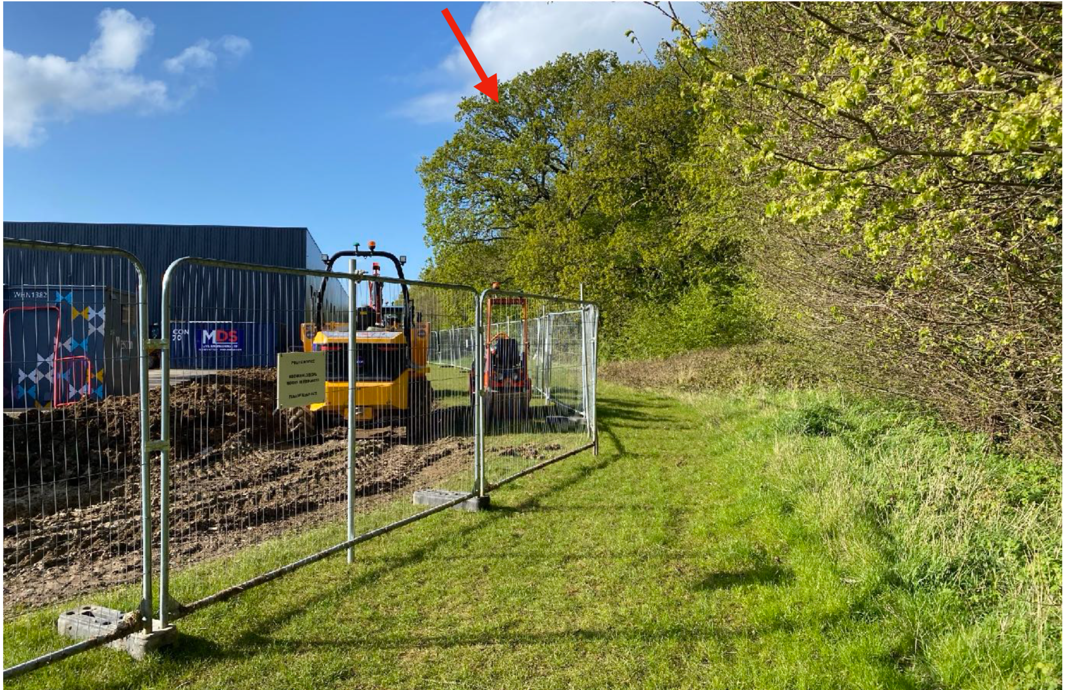
Photo 1: Fencing and heavy construction equipment well within the 15m buffer zone of Priors Wood. The ground is being extensively disturbed within RPA (Root Protection Area) including that of the veteran oak tree identified in the Arboricultural Impact Assessment as T20 (highlighted by red arrow).
