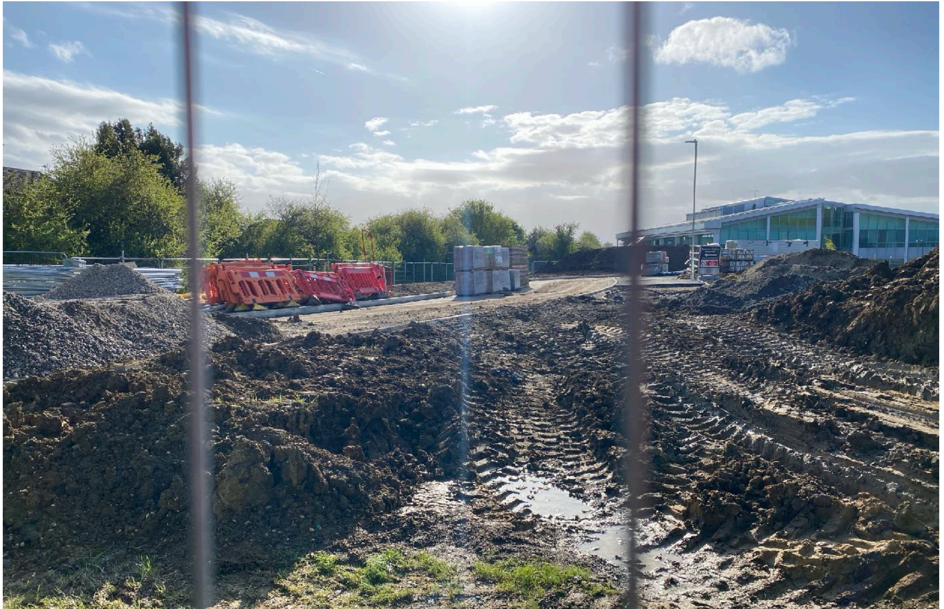
Photo 3: Section of roadway under construction in south east corner of site not shown on planning application documents. Note the heavy vehicle movements right next to Priors Wood.
