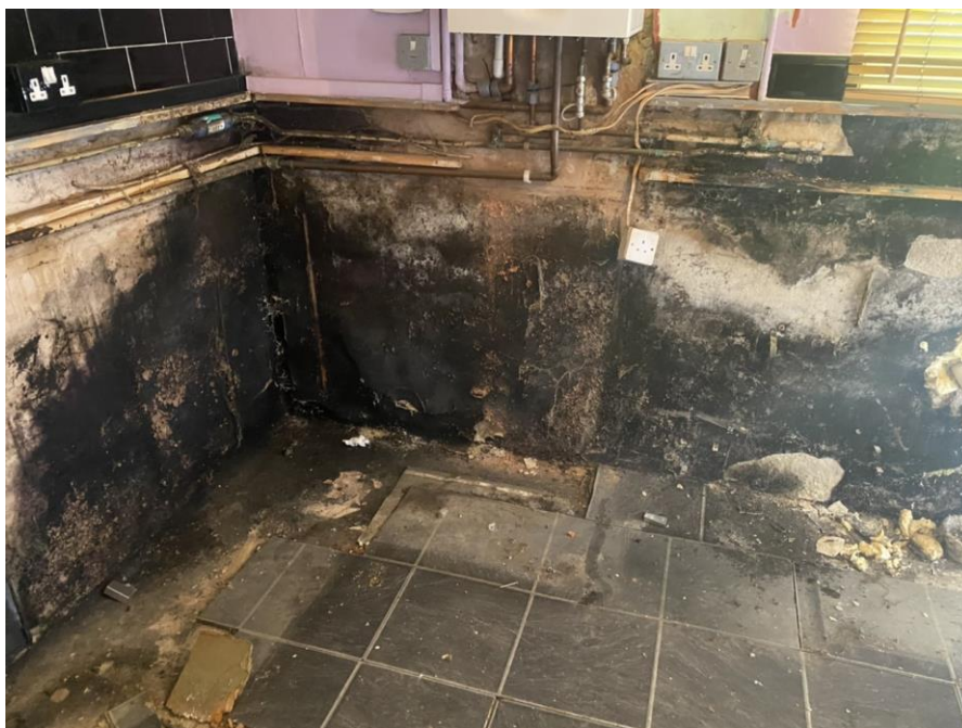
FIGURE 7 EXAMPLE OF DAMP AND MOULD PRE-RETROFIT IN HOUSE ON BROWNING AVENUE
