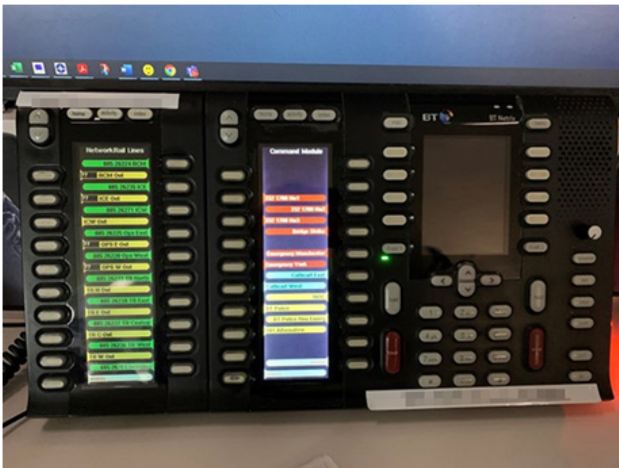
Figure 22: Telephone concentrator at the SICC (courtesy of Network Rail).
