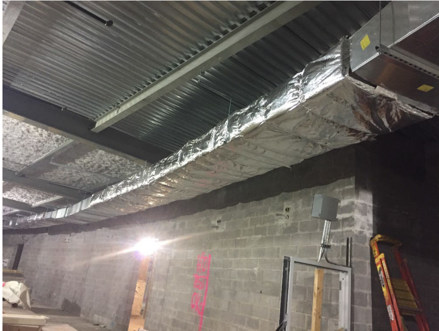
Figure 7-4 Insulation around HVAC duct work
