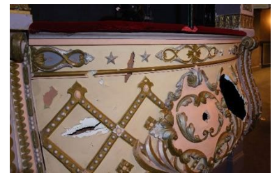
Serious damage left unrepaired: Significant damage to surfaces and some structural elements means some areas are unusable
