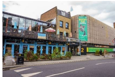
Irregular maintenance leading to paint falling away and plaster damage to frontage
