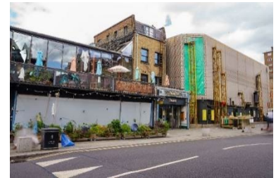
Frontage in disrepair with long-term scaffolding and wooden boarding
