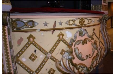
Visible wear and tear: Interior surfaces (e.g box fronts) chipped and peeling in place
