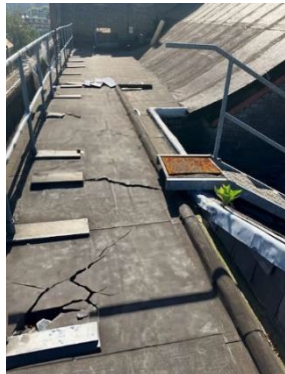
Roof irregularly inspected leading to surface cracks
