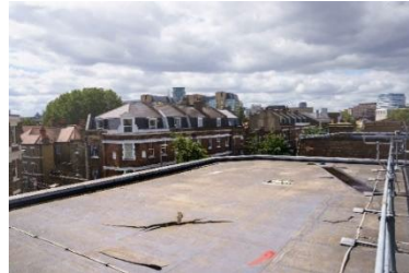
Roof irregularly inspected leading to surface cracks
