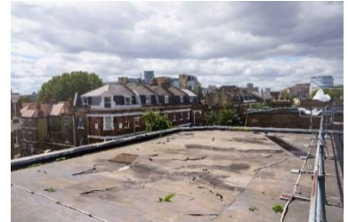
Ongoing cracks and leaks risking structural integrity of roof
