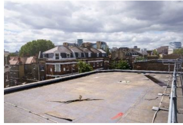
Roof irregularly inspected leading to surface cracks
