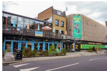
Irregular maintenance leading to paint falling away and plaster damage to frontage
