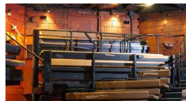
Serious damage left unrepaired: Significant damage to surfaces and some structural elements means some areas are unusable
