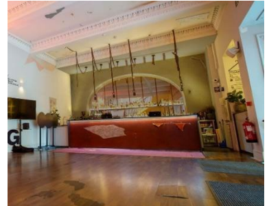
Serious damage is left unrepaired to floors, walls and ceilings
