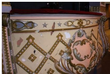
Visible wear and tear: Interior surfaces (e.g. box fronts) chipped and peeling in place
