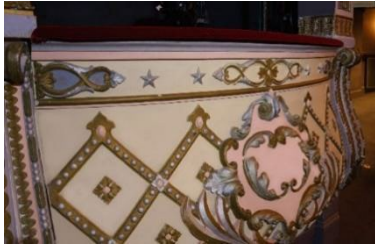
Interior surfaces (e.g box fronts) of auditorium in good condition with minimal to no marks or damage
