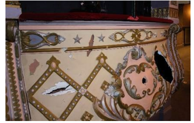
Serious damage left unrepaired: Significant damage to surfaces and some structural elements means some areas are unusable
