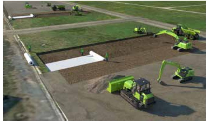
A CGI of the work that will take place on the legacy trenches
