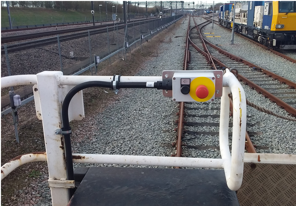
Figure 14: The new emergency stop and horn buttons on HS1 MPVs.
