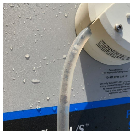
Figure 11. Sediment being pumped through tubing. This should be avoided. There may be a need to reposition the intake location [Step 7].
