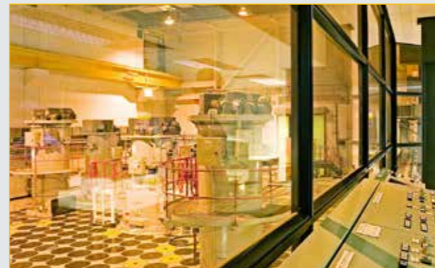
Waste Vitrification Plant
