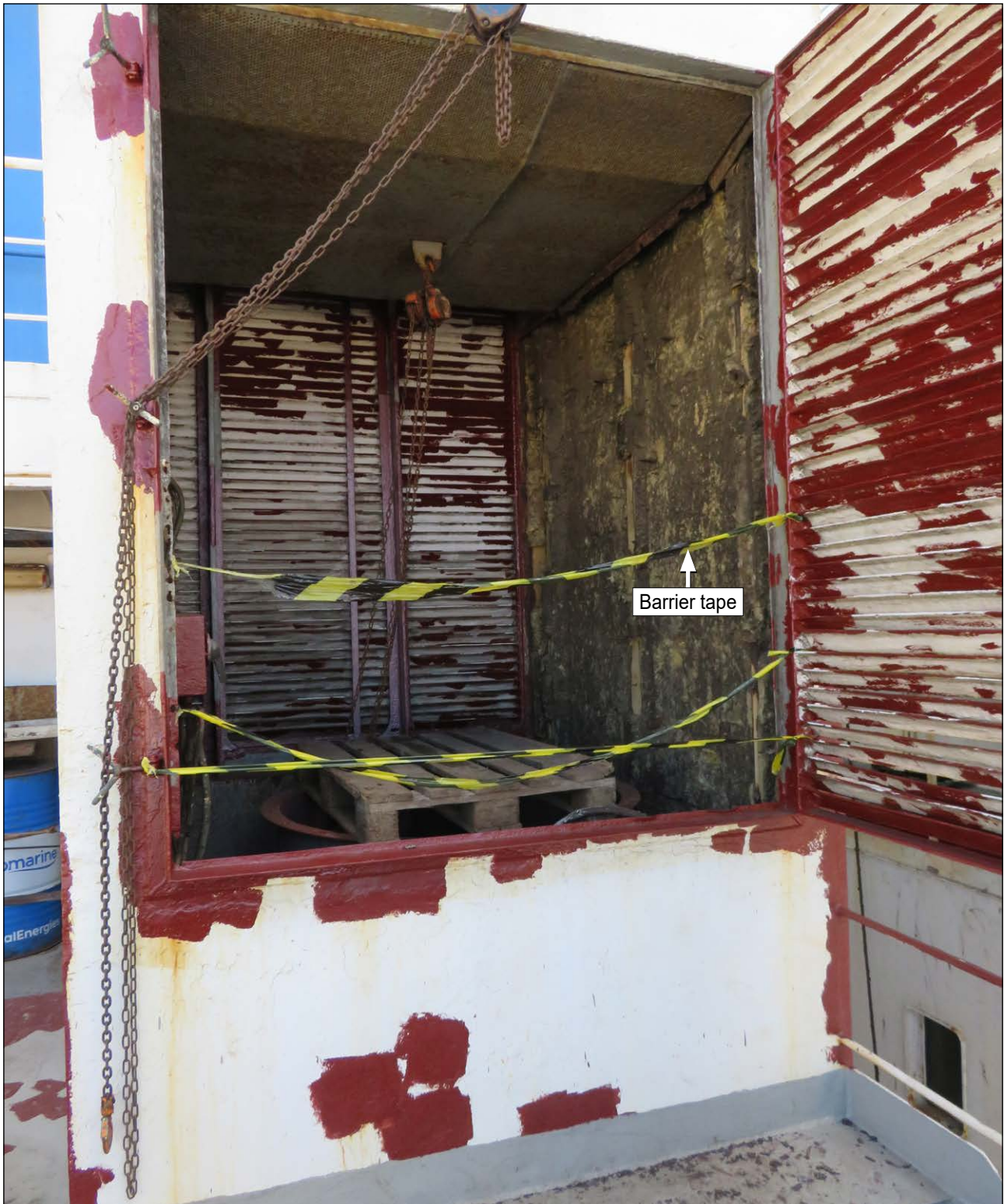
Figure 9: Barrier tape across the fan room access
