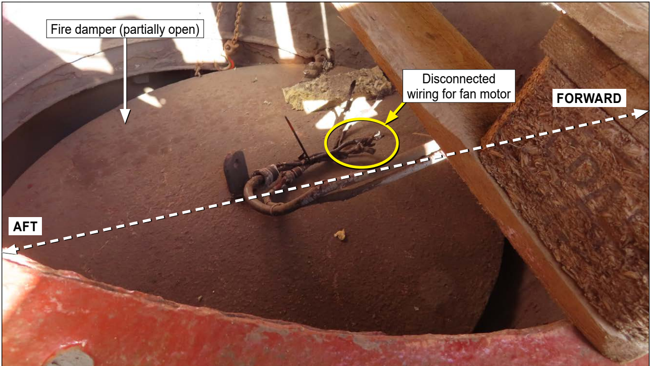
Figure 4: Starboard engine room fan pedestal fire damper
