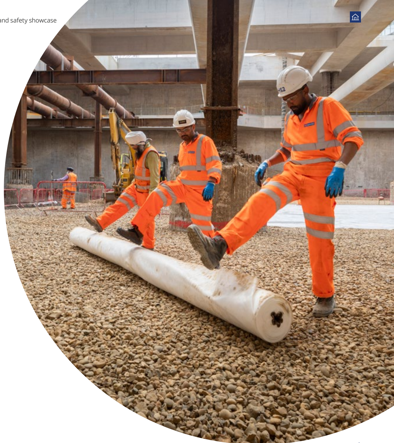
Front cover image: HS2 worker at Curzon Street. Right: Workers placing waterproofing layers in base level at Old Oak Common.
