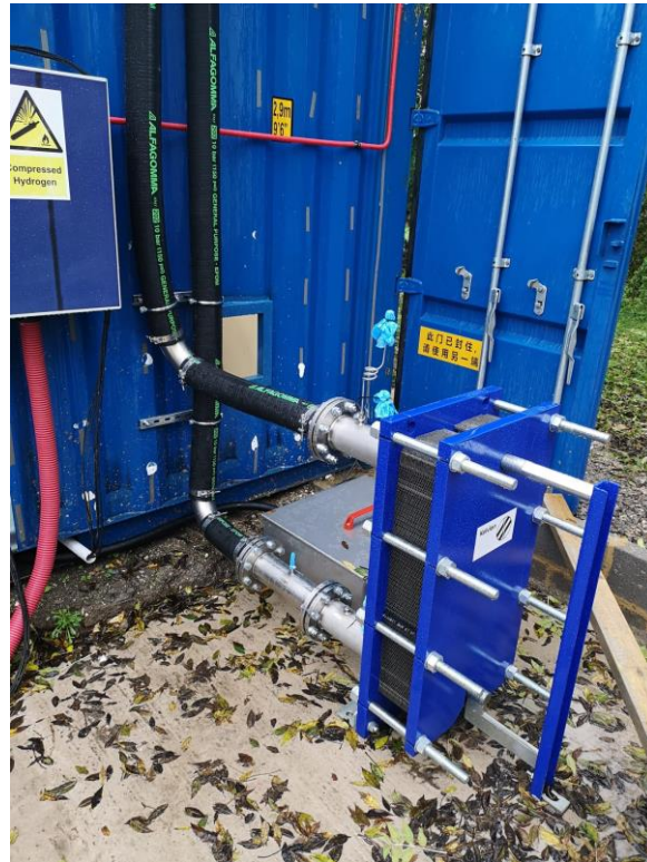
Figure 16 - Condenser system – Kelvion Plate & Gasket Heat exchanger and Nixon Flowmeter
