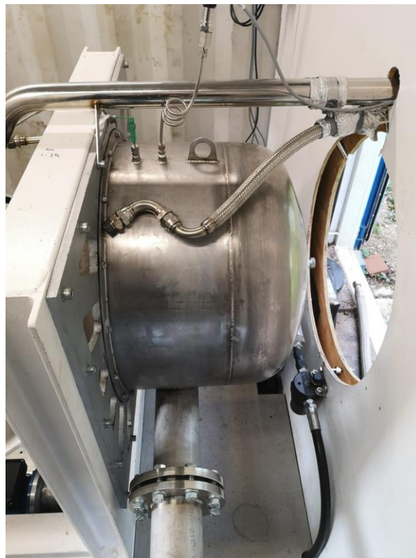
Figure 15 - Condenser System – Plenum
