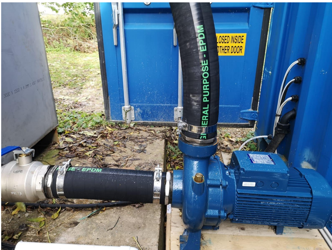
Figure 17 - Condenser system- High flow coolant Pump
