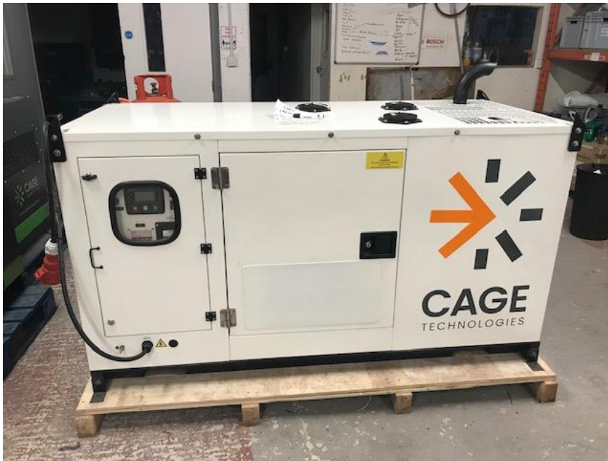
Figure 10 CAGE 15PG generator
