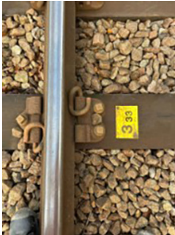
Figure 13: Railhead condition near the site of the accident on 21 November. Image also shows a chainage marker plate provided at regular intervals along the Island Line (courtesy of South Western Railway).
