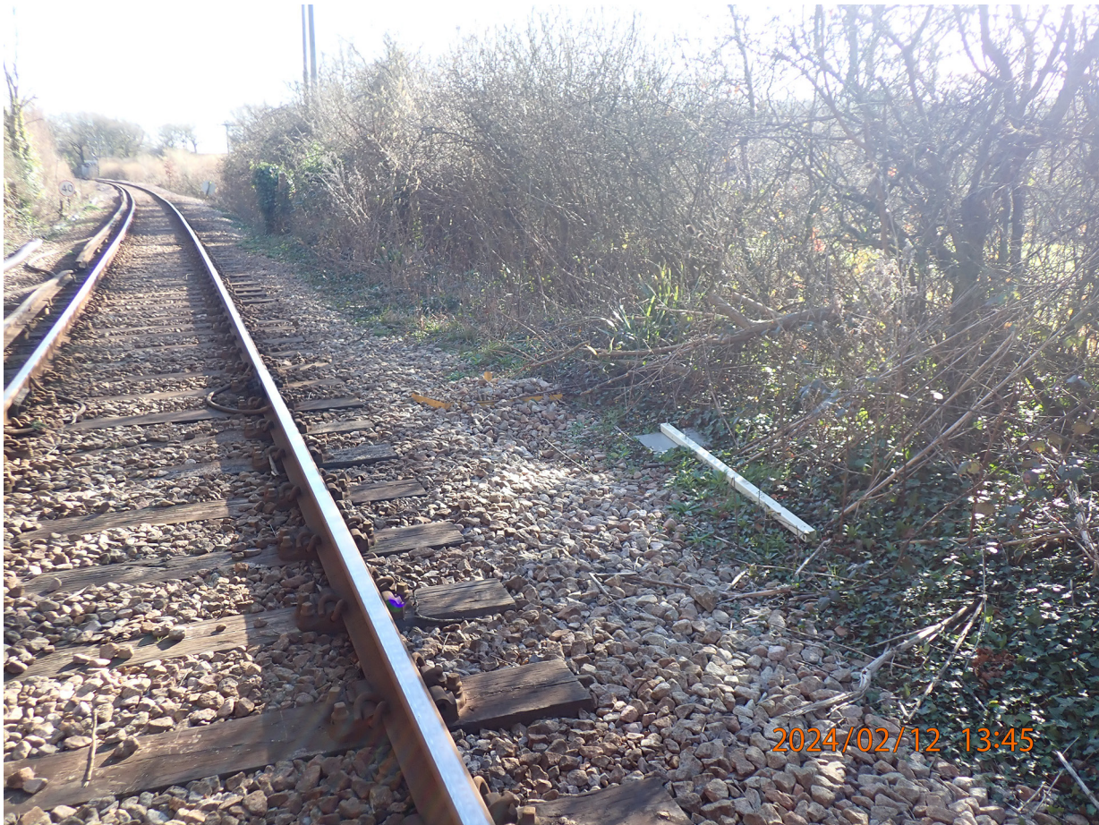
Figure 12: Location of accident looking south.
