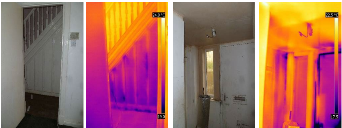
Figure 3-4 Air entering the front and rear halls from the cellar and directly from outside
