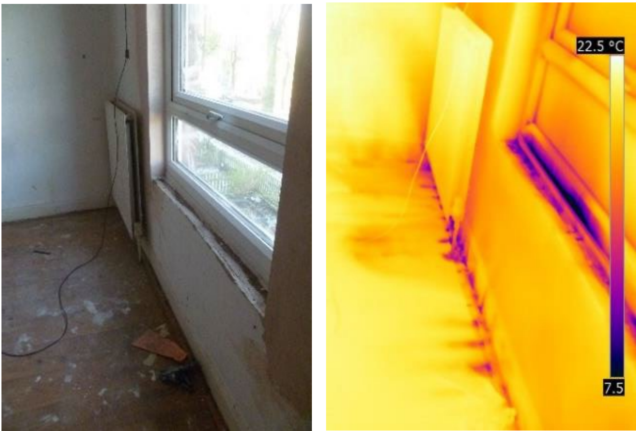
Figure 3-24 Failing mastic sealant at the unfinished plaster around the window in Bedroom 2
