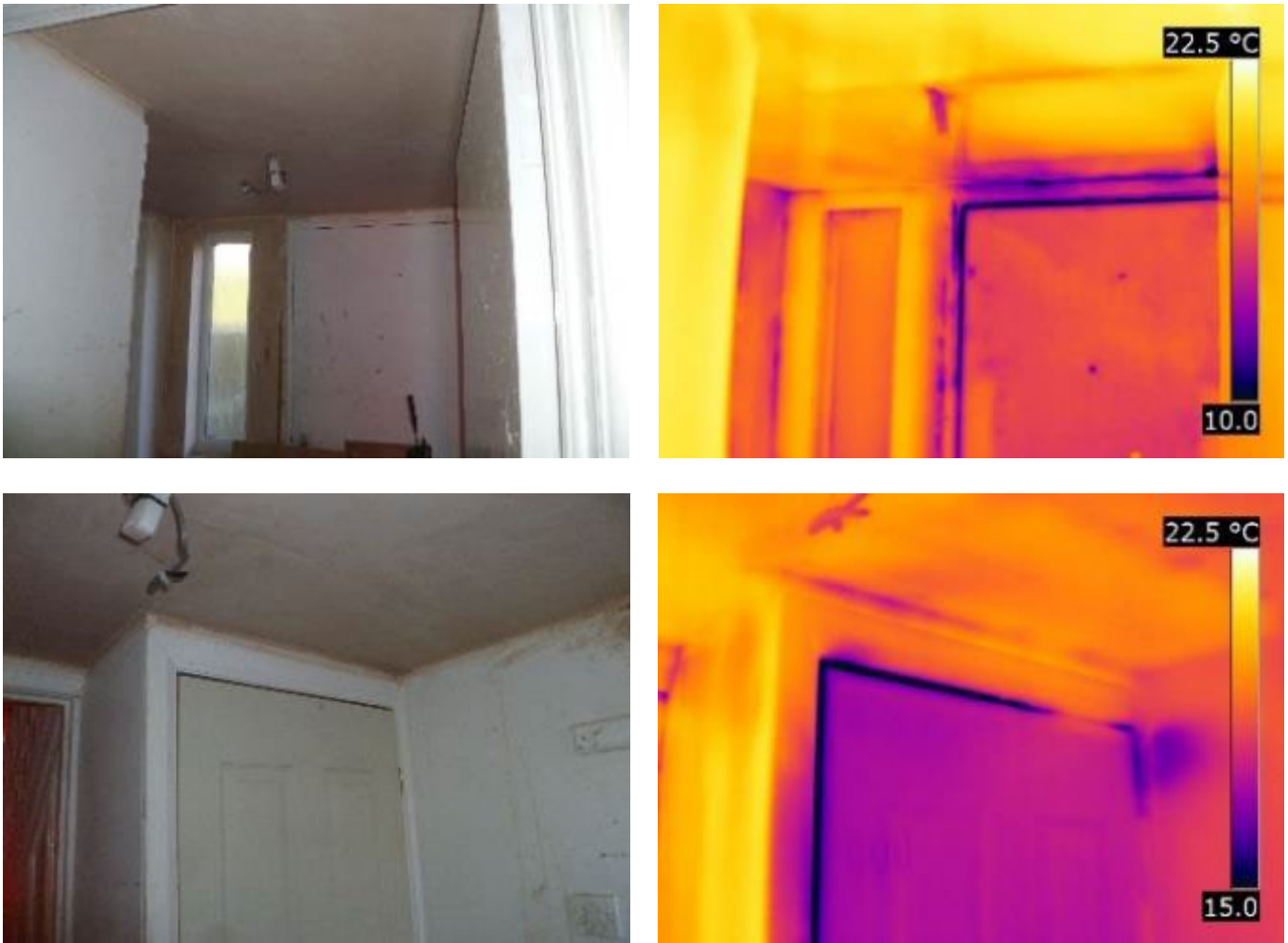
Figure 3-20 The rear (top) and cellar (bottom) doors showing air leakage
