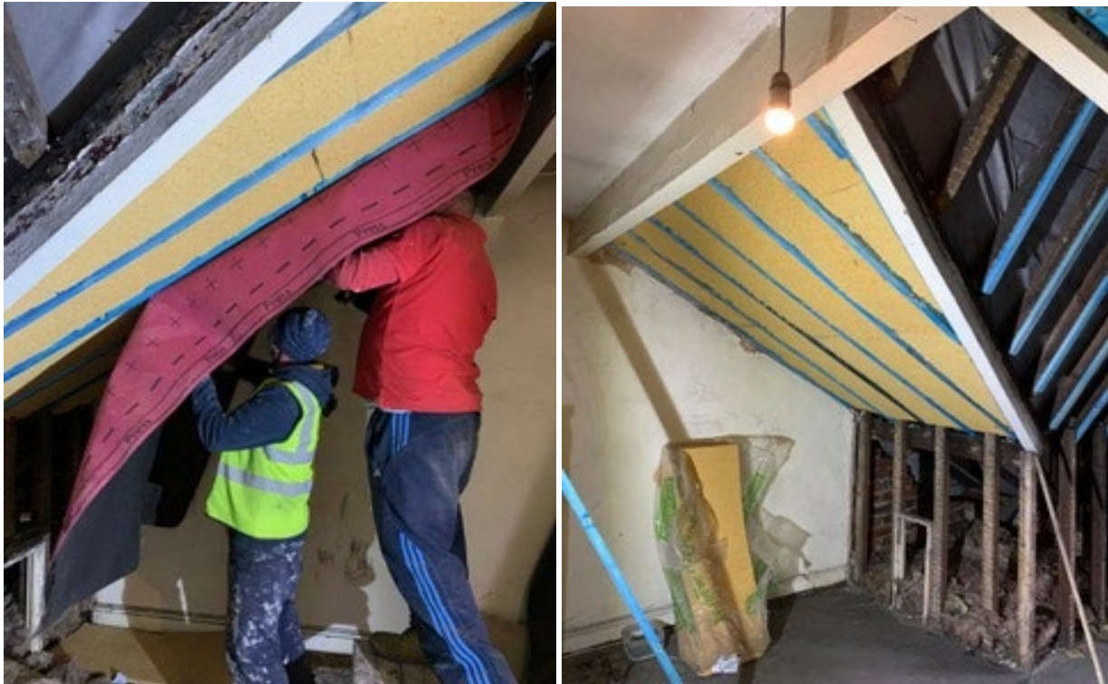
Figure 3-34 Installation of new breathable moisture membrane and additions to roof timbers (blue) to accommodate the extra thickness of the insulation
