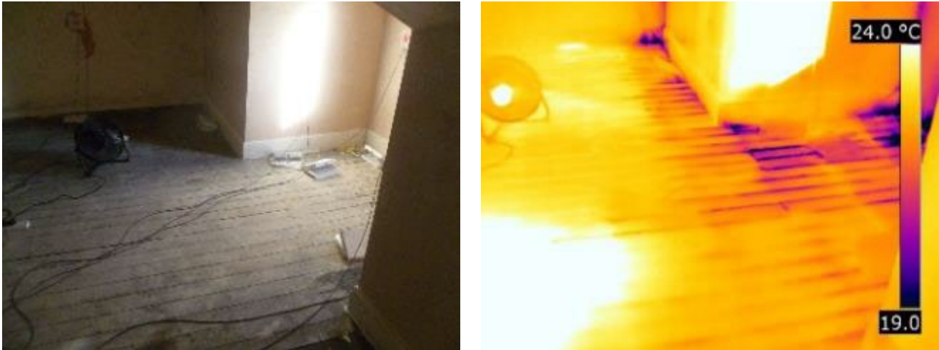
Figure 3-26 Air leakage under the floor from a boxed-in airing cupboard
