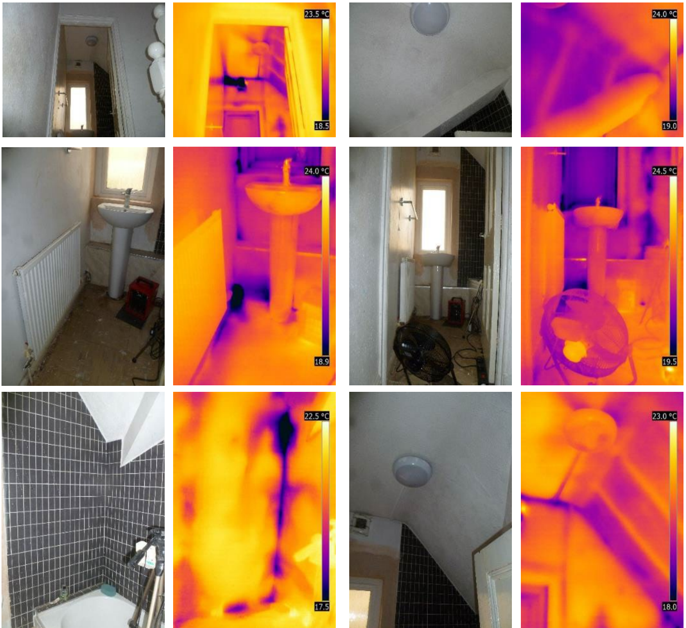
Figure 3-10 The second floor bathroom showing both direct and indirect air leakage
