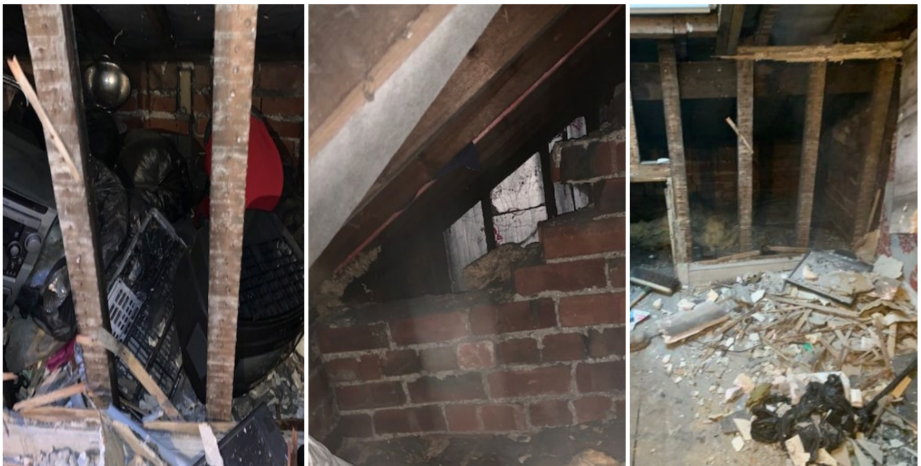
Figure 3-33 Debris behind knee walls (left), missing party wall brickwork between dwellings in eaves (middle) and substantial waste generated by the removal of existing surfaces (right)
