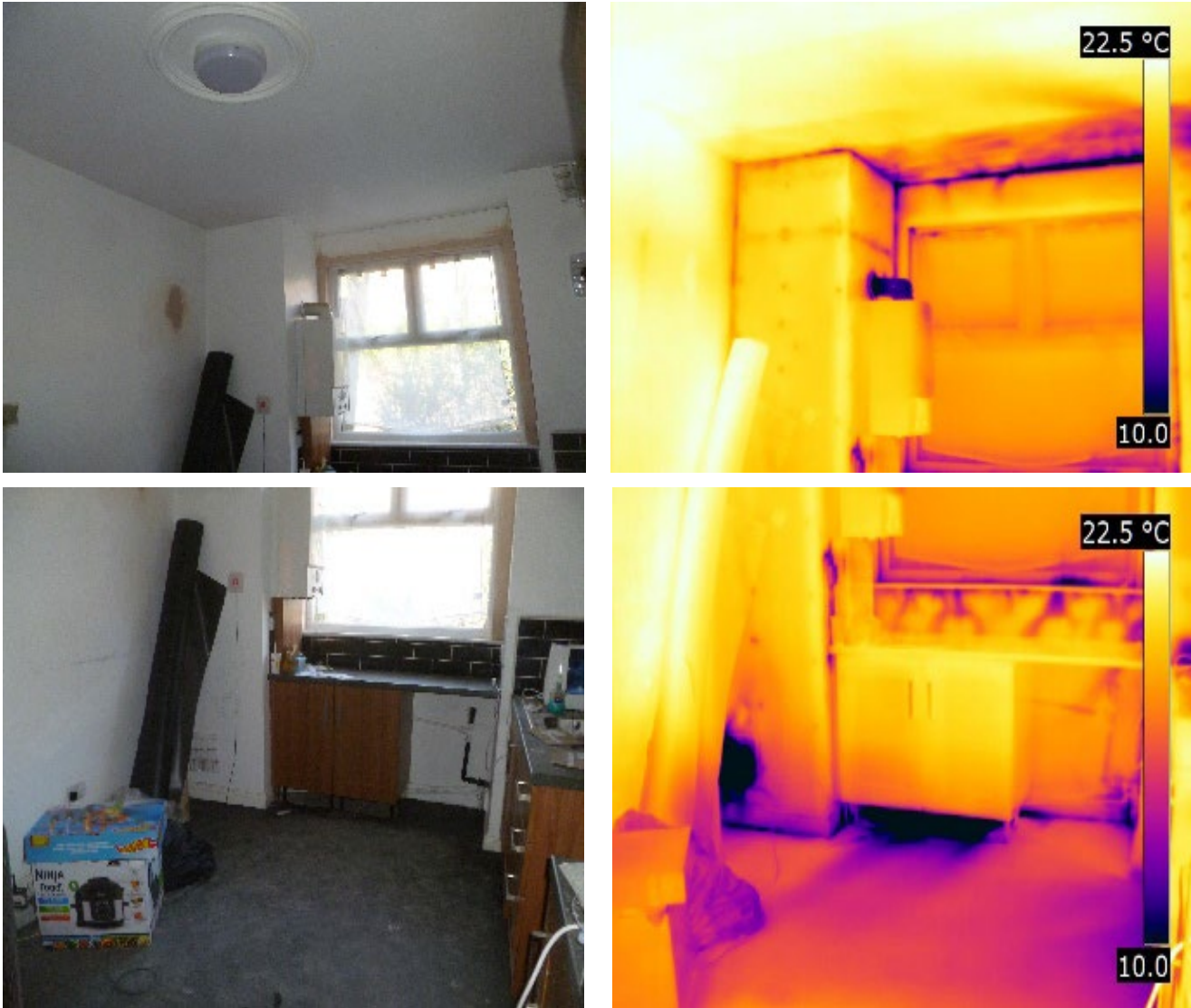
Figure 3-18 Thermographic detection of leakage at the kitchen bay
