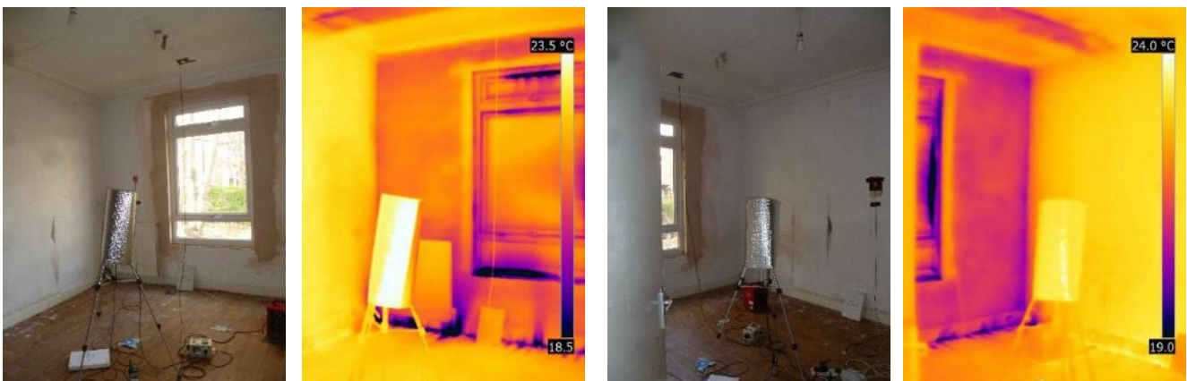
Figure 3-7 Direct air leakage in the front bedroom at the floor junction with the external wall and at the window
