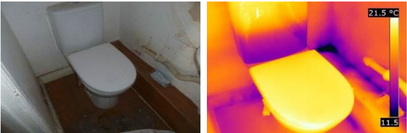
Figure 3-22 Un-adhered mastic sealant on the new boxing in the WC
