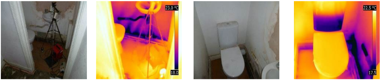
Figure 3-5 Infiltration at the first floor WC
