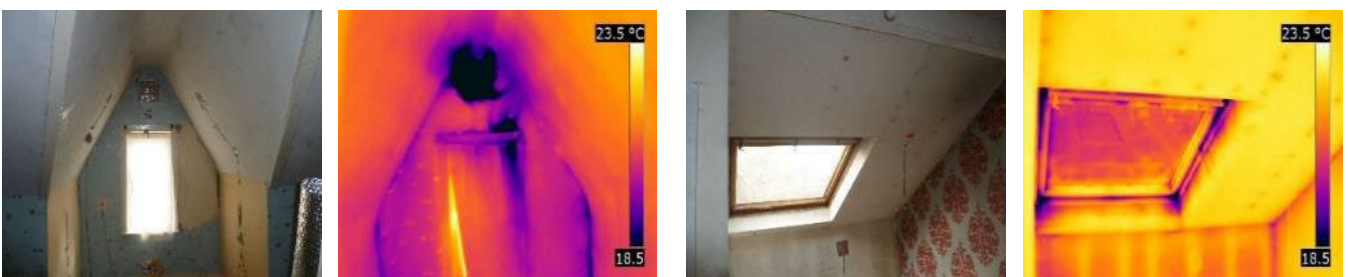
Figure 3-14 Air leakage at the windows in the front and rear bedrooms, and around the vent above the front bedroom window
