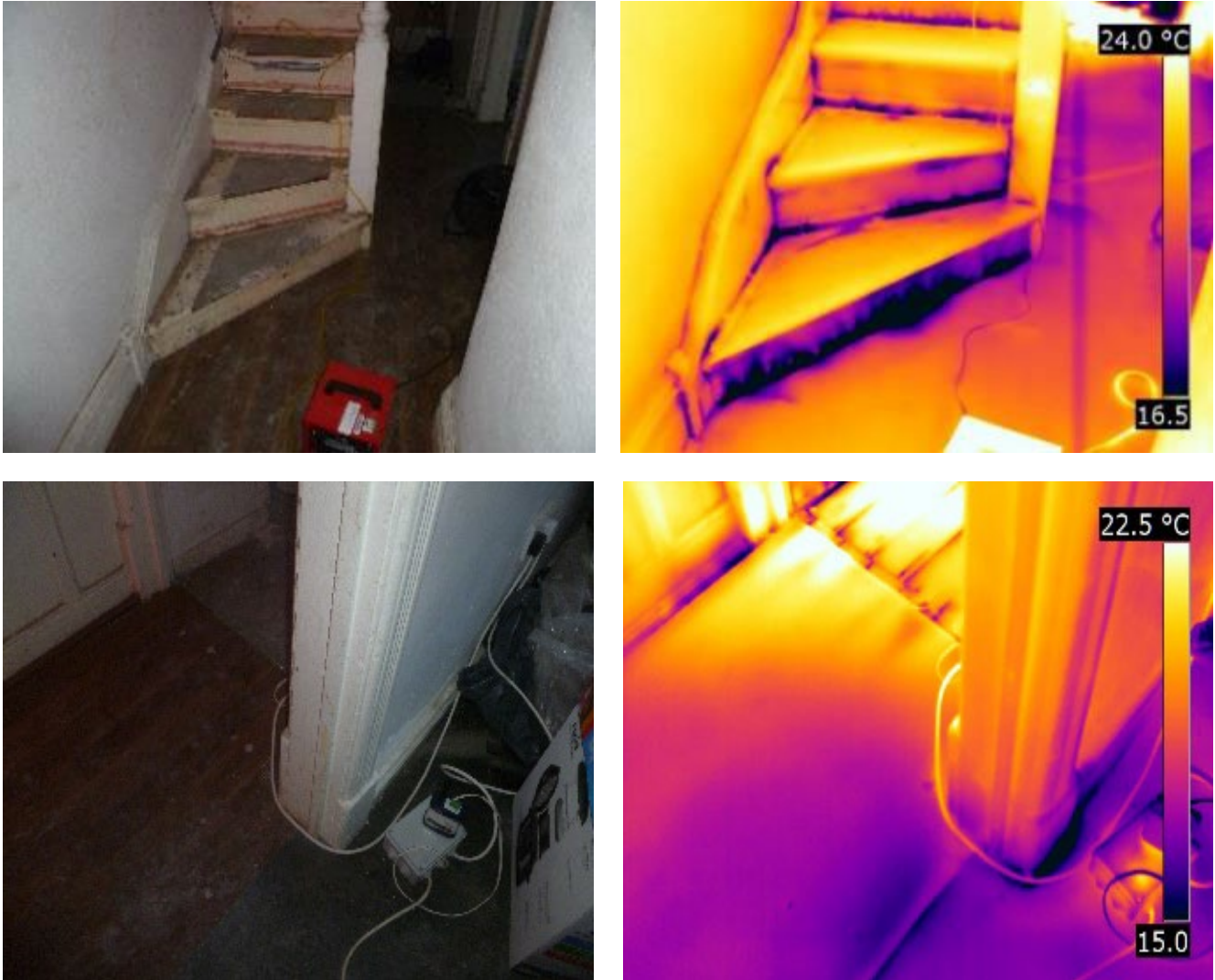
Figure 3-19 Air movement up from the cellar near the centre of the house
