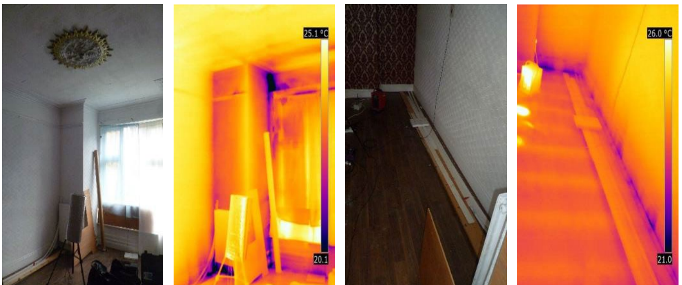
Figure 3-2 Air leakage in the living room around the bay window and ground floor perimeter
