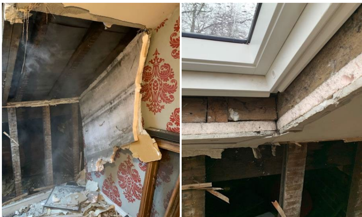
Figure 3-35 Existing insulation found installed in the room-in-roof sloping ceiling
