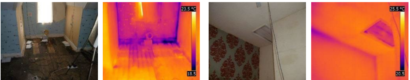
Figure 3-13 Direct air leakage in the front bedroom at the external wall junction with the floor and around the loft hatch
