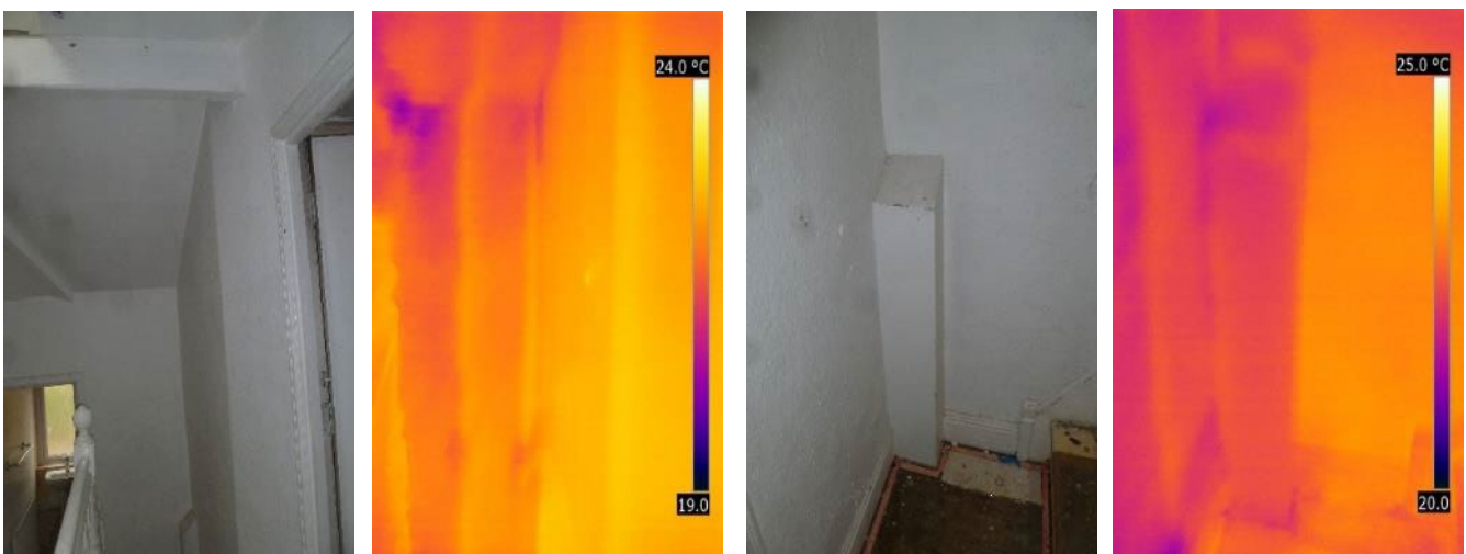
Figure 3-9 The second floor landing with cooler air being drawn through partition wall voids
