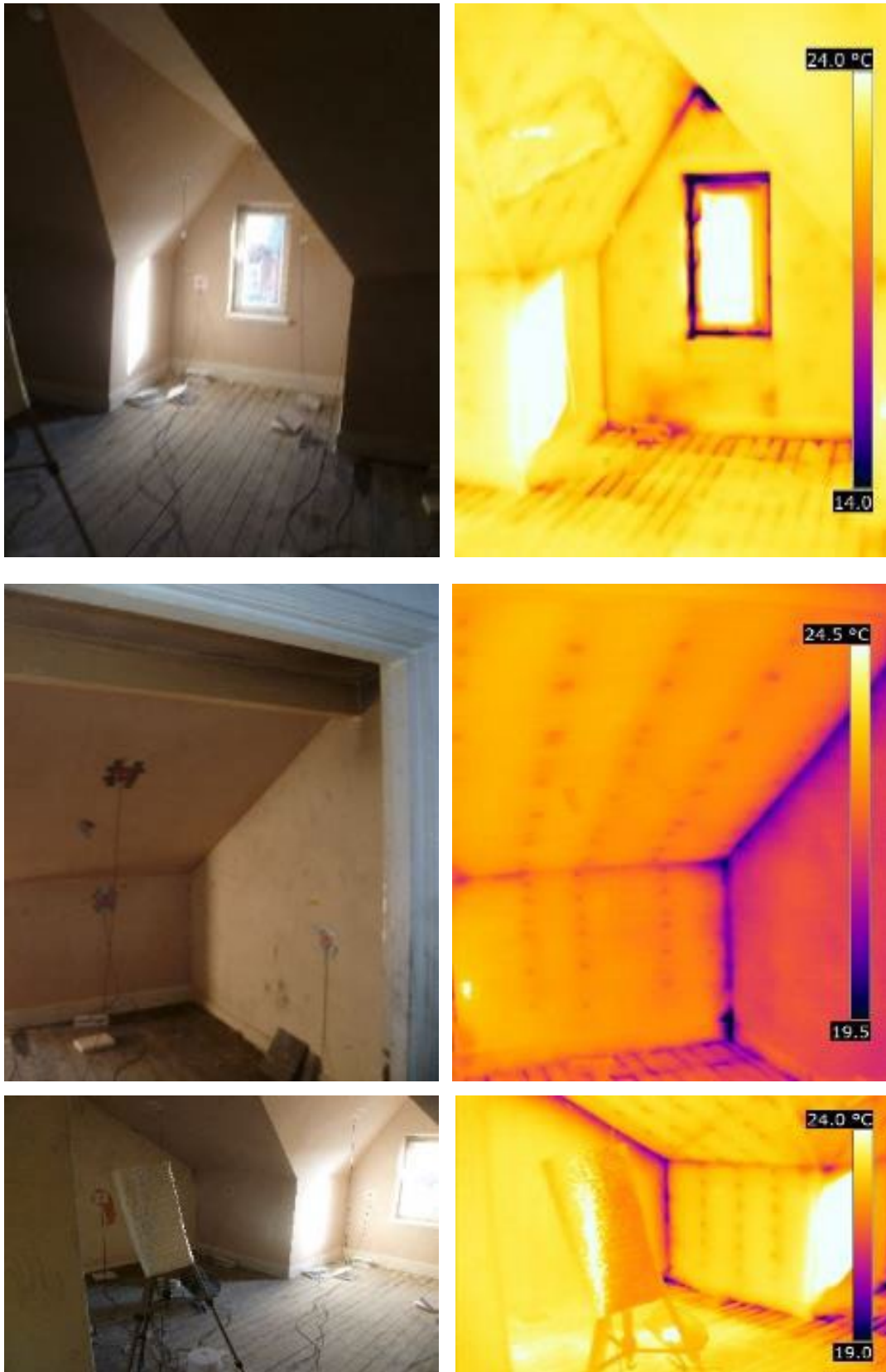
Figure 3-25 Air leakage through cracks in plaster and failed mastic seals at interfaces between elements in Bedroom 3 under depressurisation immediately following coheating
