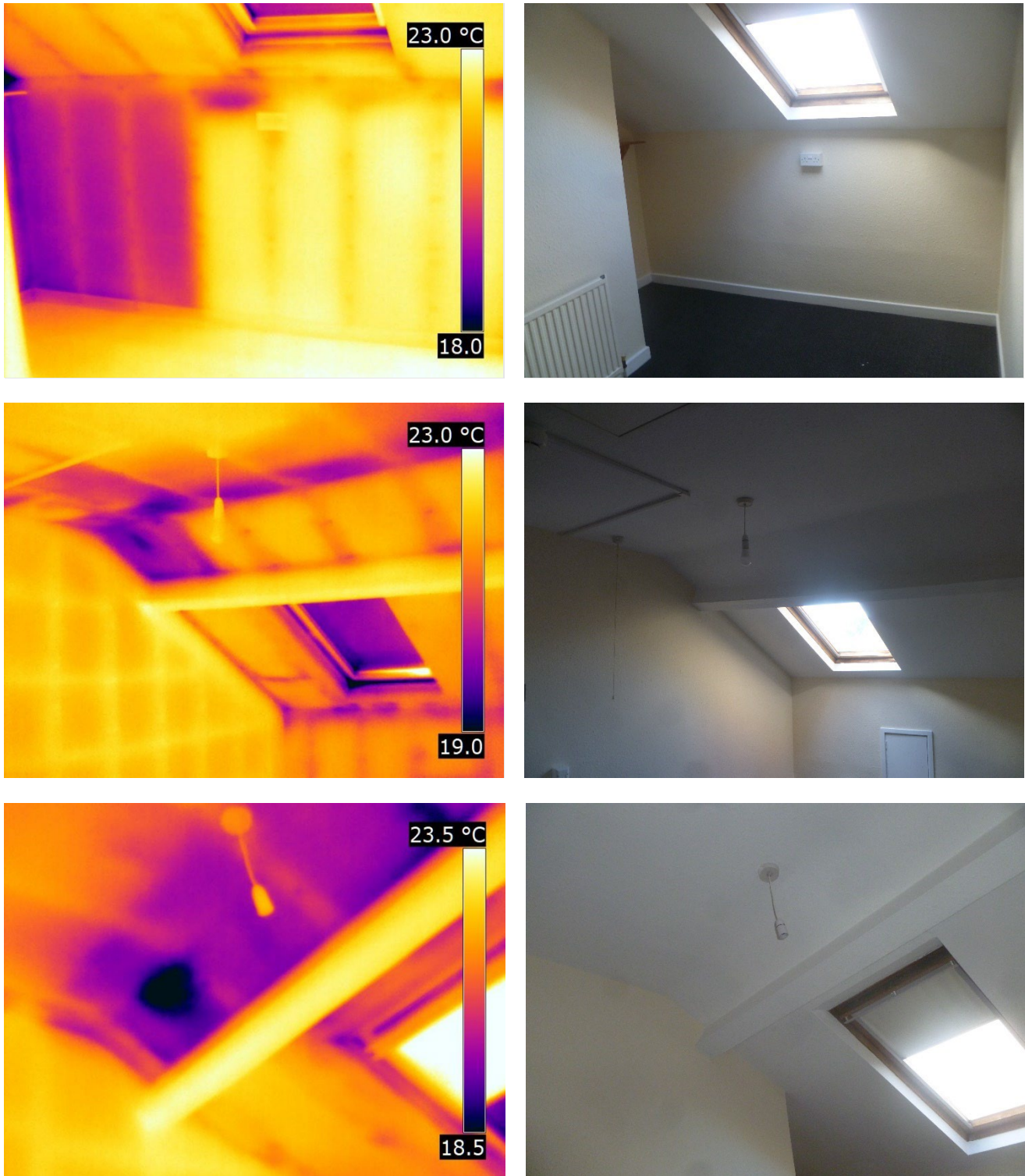
Figure 3-30 Discontinuities around complex geometries in room-in-roof pre-retrofit causing cold bridging resolved post-retrofit
