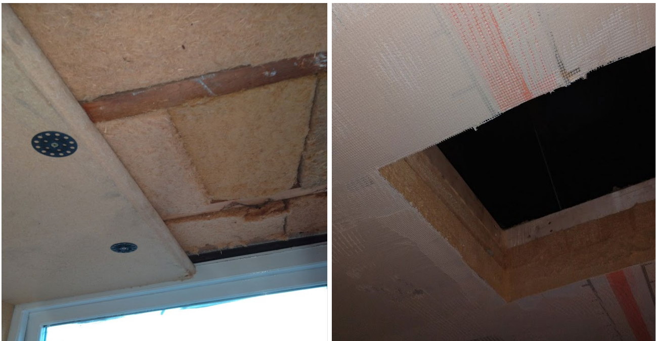
Figure 3-29 Reduction in ceiling height caused by the addition of wood fibre insulation
