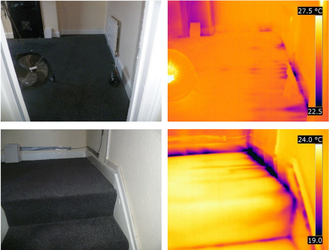
Figure 3-10 Infiltration around intermediate floor and stair perimeters
