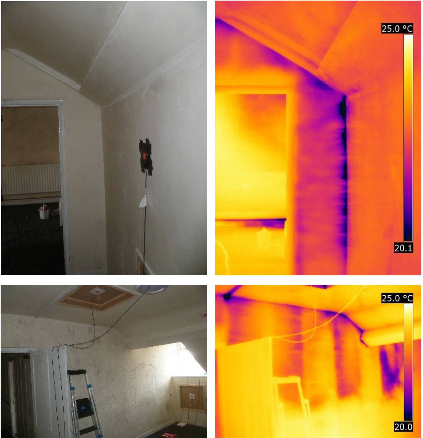
Figure 3-15 Indirect air leakage into the second floor partition wall voids in 07LT
