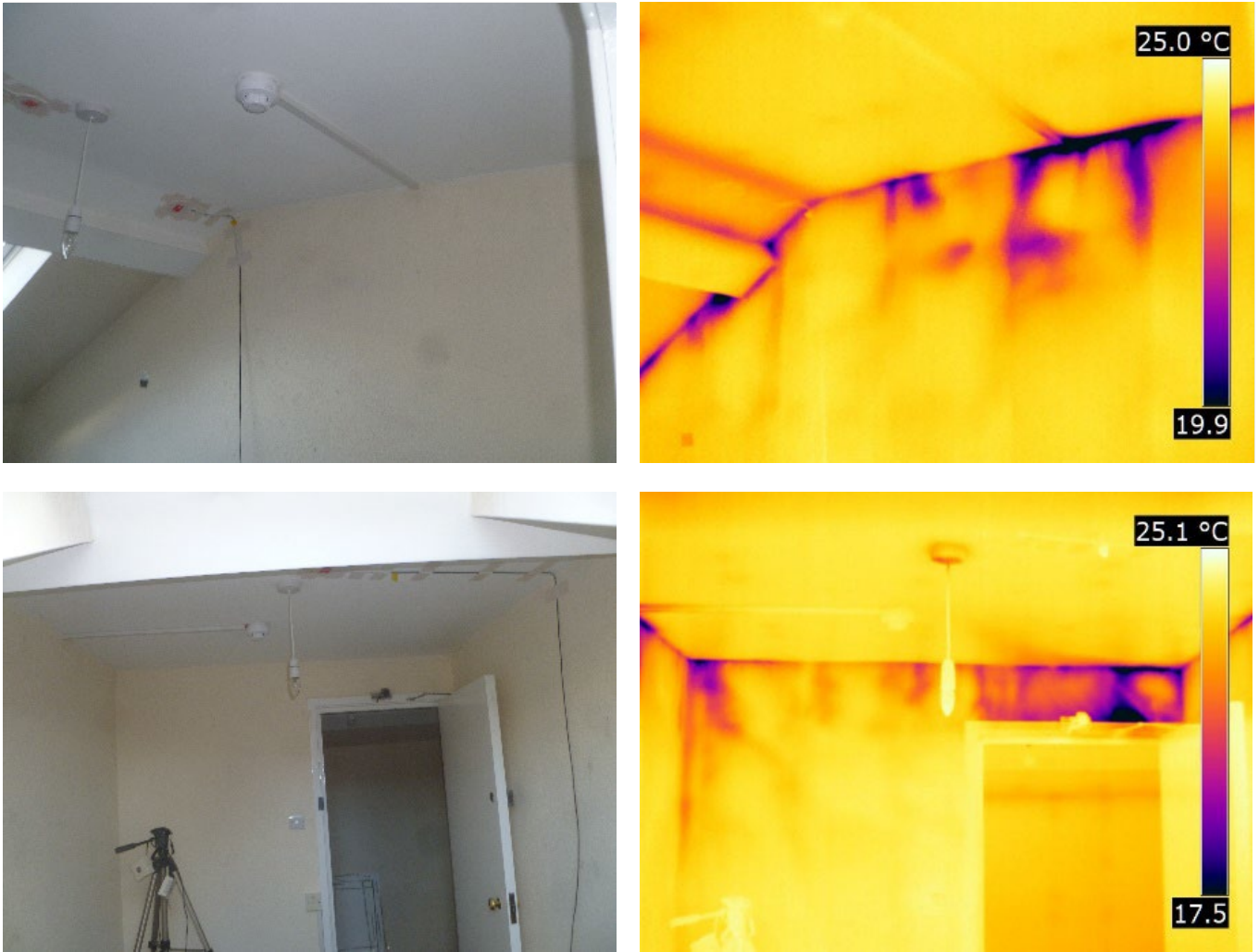
Figure 3-16 Indirect air leakage into the second floor partition wall voids in 09LT
