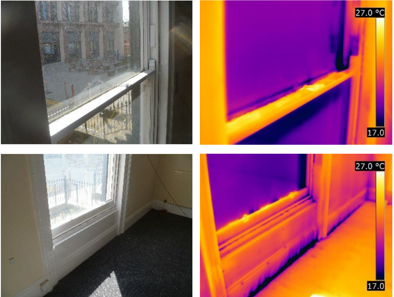
Figure 3-22 Front room in 07LT showing reduced air leakage at meeting rails and lower sash
