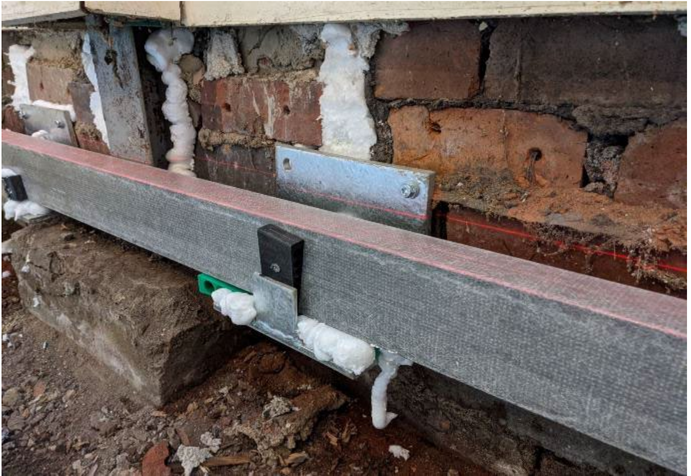
Figure 3-21 Insulated floor supports to reduce thermal bridging at the ground floor to wall junction
