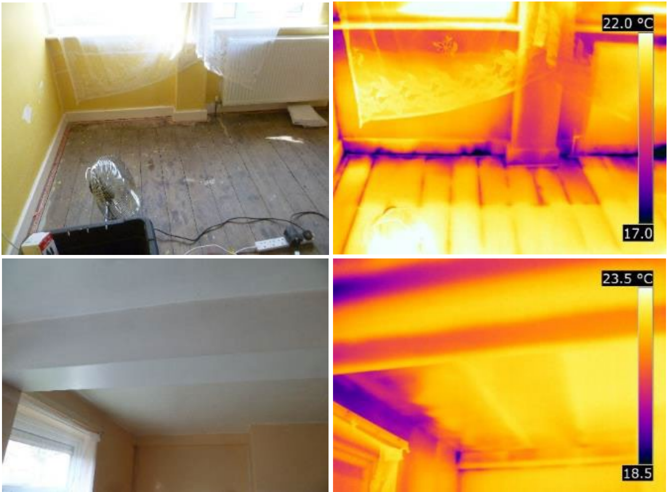
Figure 3-6 Indirect air leakage via the intermediate floor void from above (top) and below (bottom)
