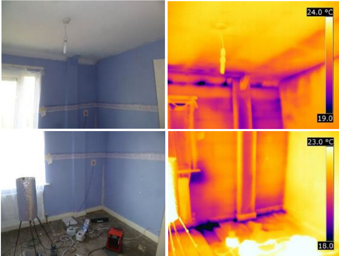
Figure 3-8 Boxed-in pillar in Bedroom 2 viewed from inside under depressurisation as cold air is drawn down into the habitable space from the loft space
