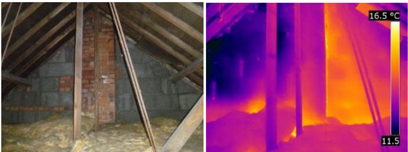
Figure 3-11 The cavity party wall in the loft, showing a potential cavity party wall bypass heat loss mechanism in effect
