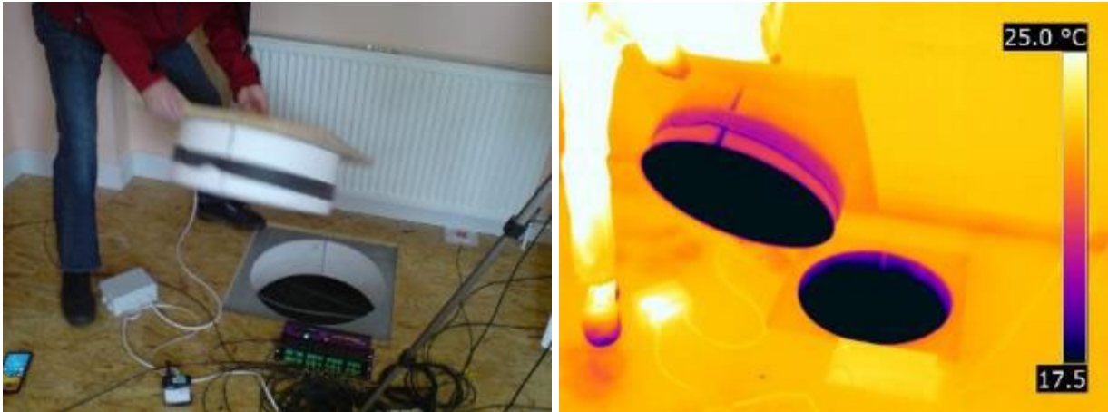
Figure 3-14 Temporary removal of the sub-floor void access hatch in the post-retrofit living room floor, illustrating the thermal gradient through the replacement flooring
