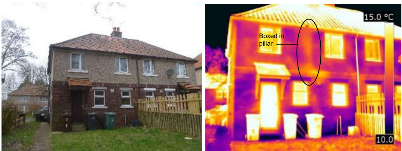
Figure 3-9 Boxed-in pillar in Bedroom 2 viewed from outside under natural conditions showing warm air from the habitable space travelling through the wall cavity to the loft space
