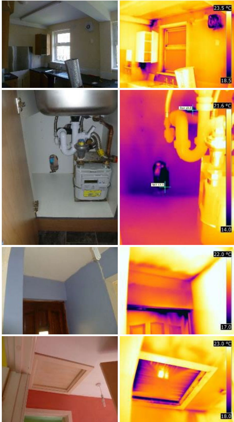
Figure 3-5 Direct air leakage at service penetrations, the rear external door and loft hatch
