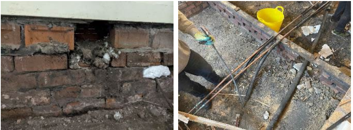
Figure 3-23 Floor void vents blocked and water pipes not effectively insulated pre-retrofit
