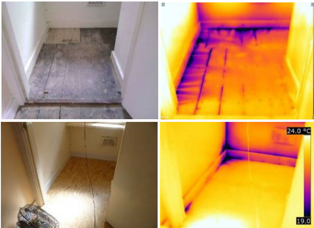
Figure 3-3 The living room cupboard with original floor (top) and replacement floor (bottom)
