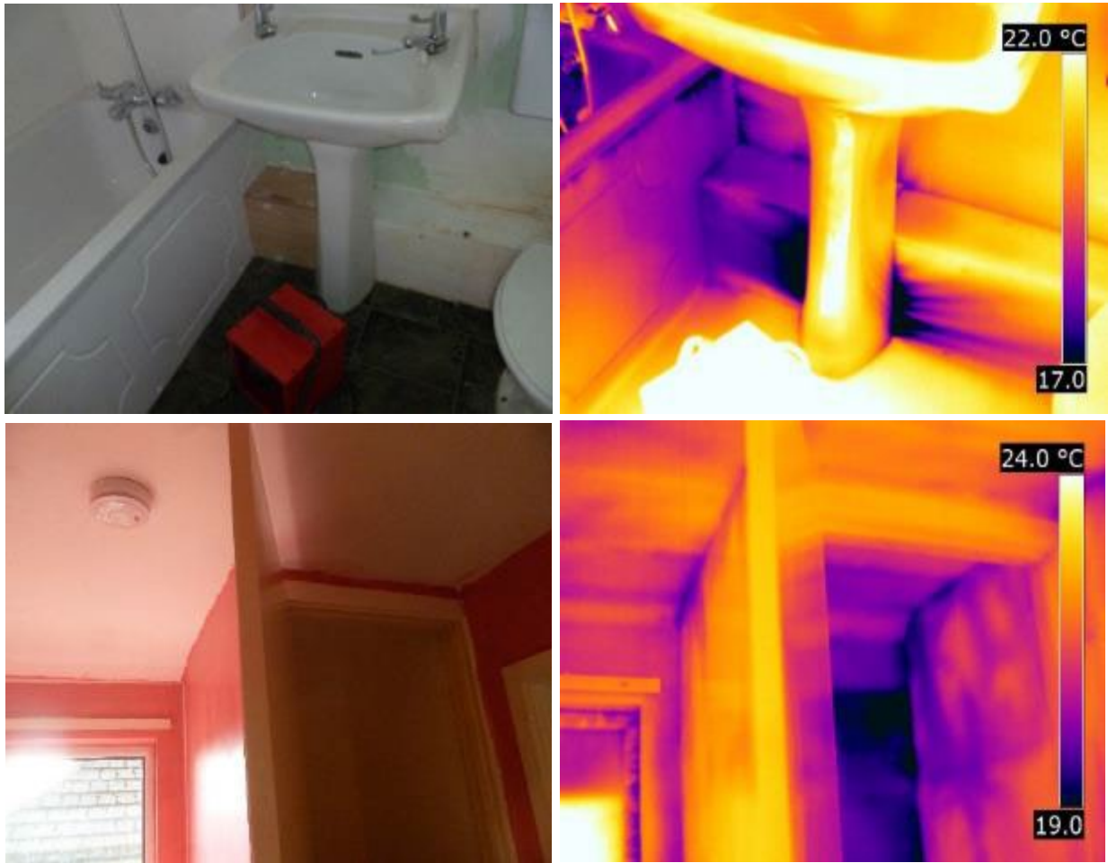
Figure 3-7 Indirect air leakage via boxed in pipework in the bathroom (top) and the airing cupboard wall (bottom)
