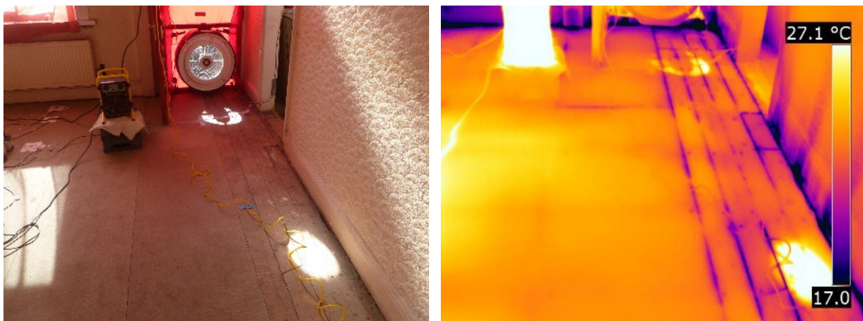
Figure 3-9 Infiltration around the perimeter of the suspended timber ground floor after XPS retrofit during depressurisation
