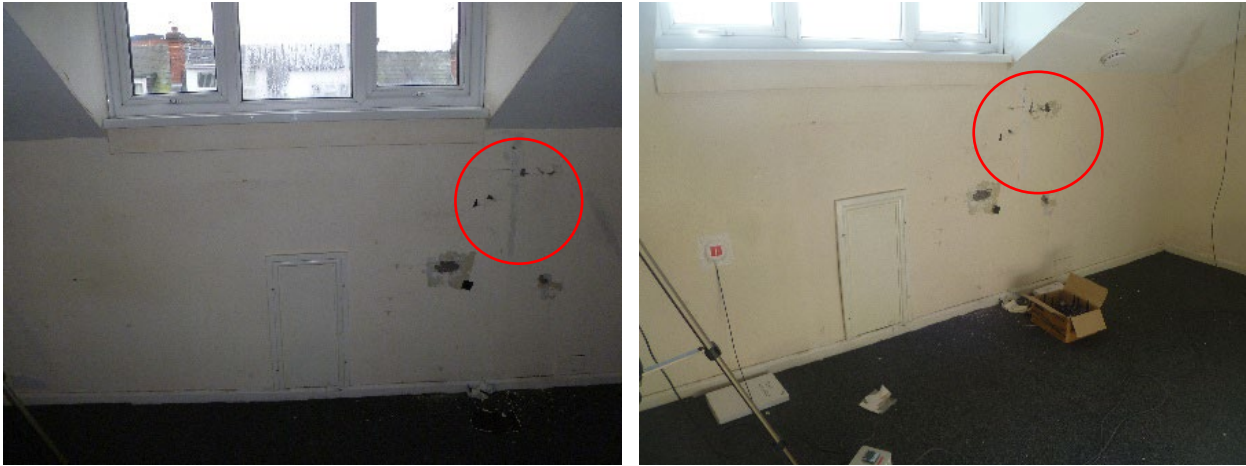
Figure 3-10 Deteriorating fabric causing worsening infiltration between first test (left) and final test (right)
