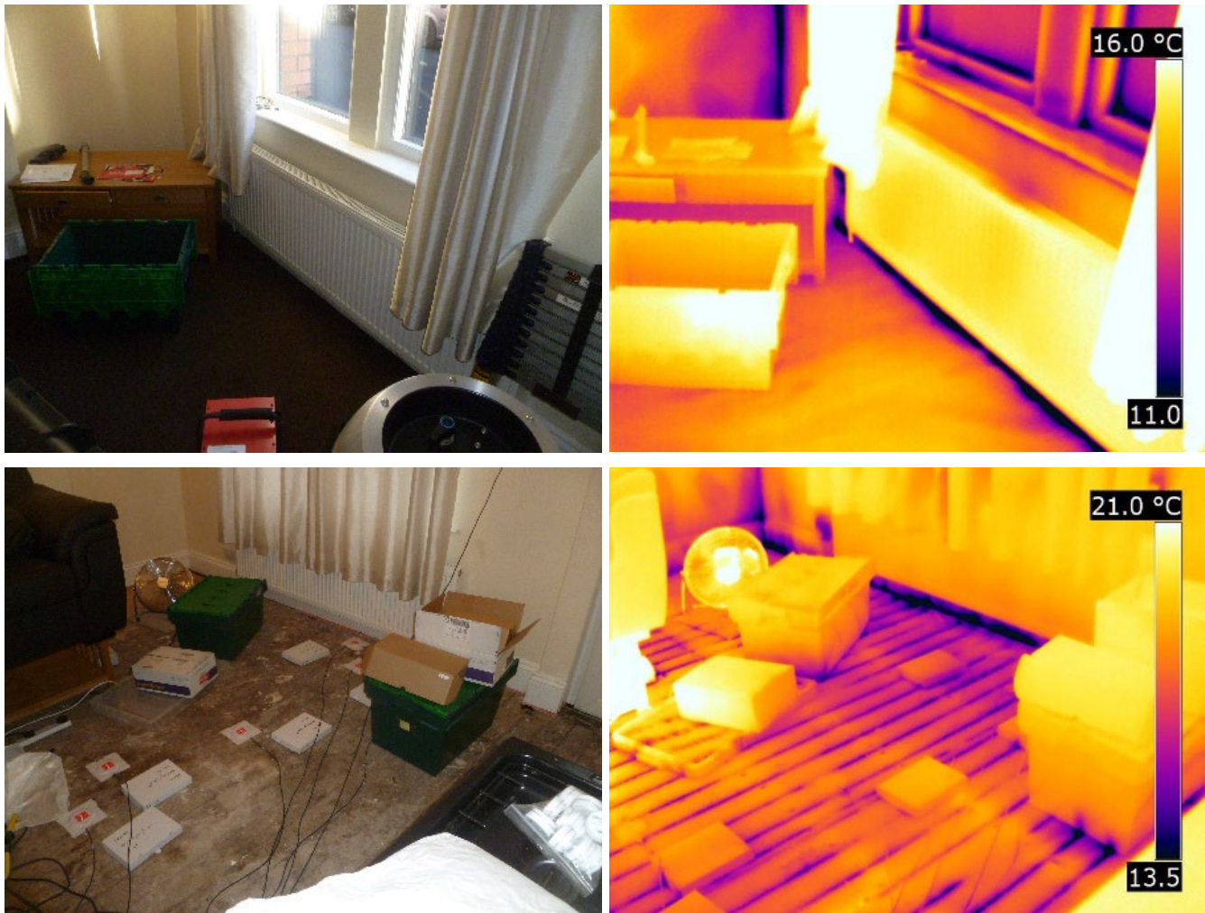
Figure 3-6 52NP Living Room showing limited air infiltration through the ground floor with carpets (top), and greater infiltration after carpets were removed (bottom) during depressurisation
