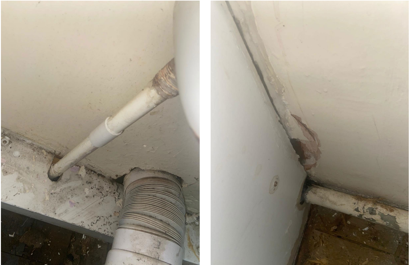
Figure 3-5 Unsealed WC waste pipe (left) and boxed-in pipework requiring destructive investigation to facilitate sealing (right)
