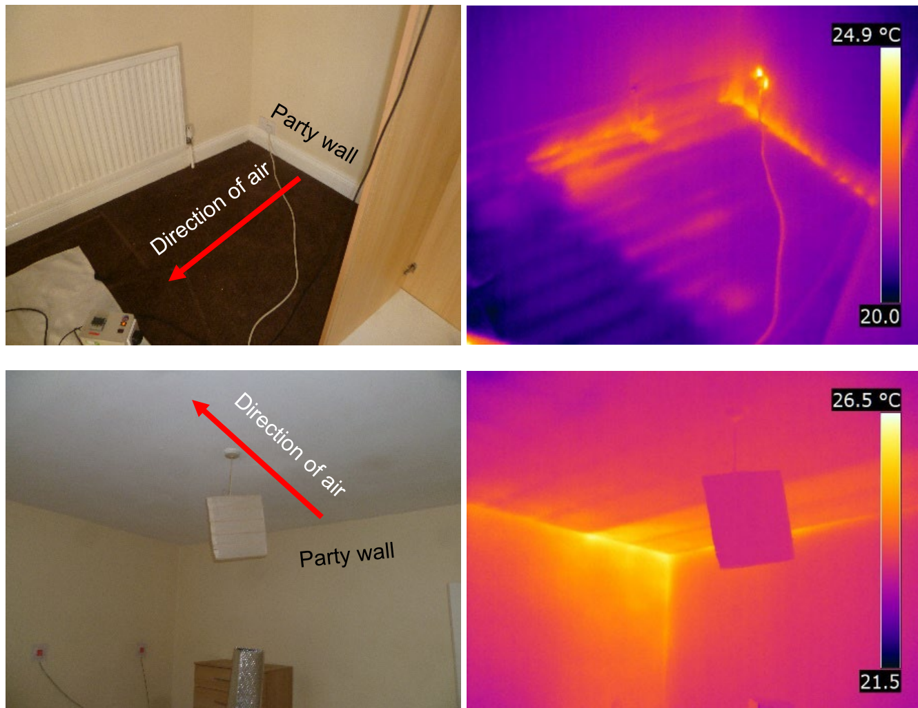
Figure 3-4 Warm air from neighbouring dwelling entering 54NP via first floor intermediate floor (top) and second floor intermediate floor (bottom)
