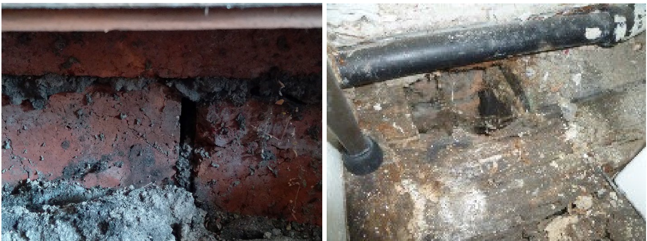
Figure 3-3 Mortar gaps and cracks in intermediate floor party wall brickwork
