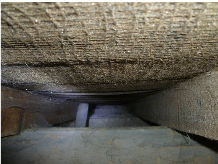
Figure 3-13 Image showing no insulation in skeilings
