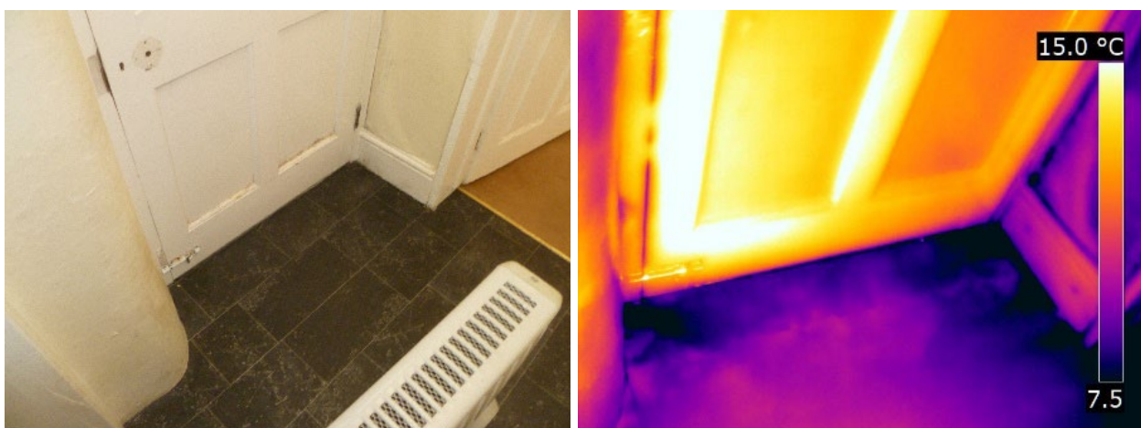
Figure 3-1 Base case infiltration around front door during depressurisation
