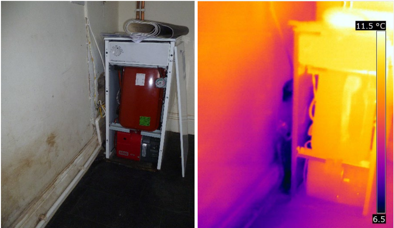
Figure 3-2 Base case infiltration through unsealed service penetrations attached to the boiler during depressurisation
